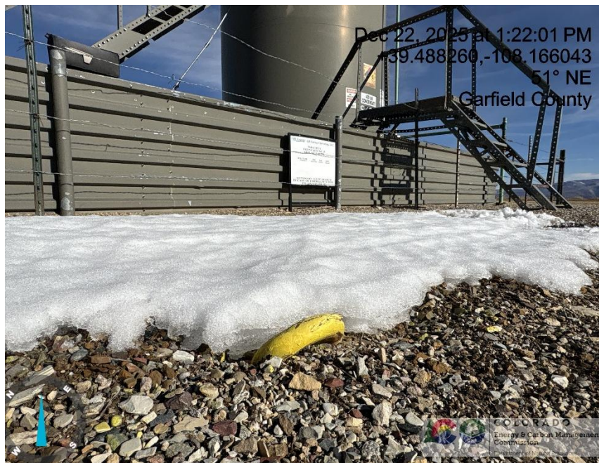
Photo # 5087 Same unmarked deadman
