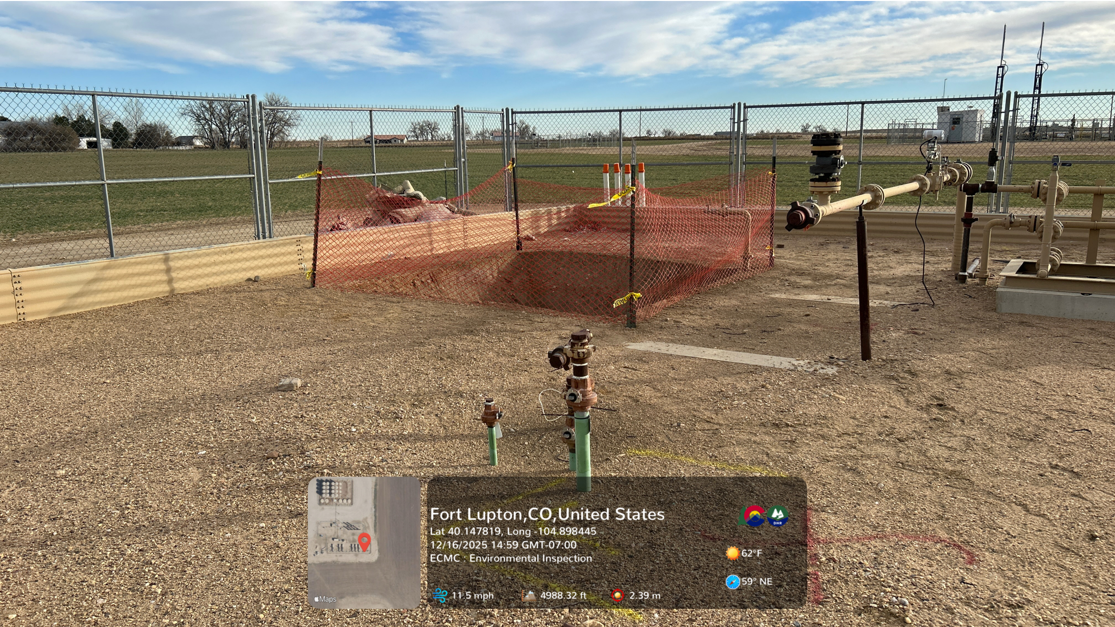
Looking at the spill location. An excavation is open at the spill location. Orange construction fencing surrounds the open excavation.
