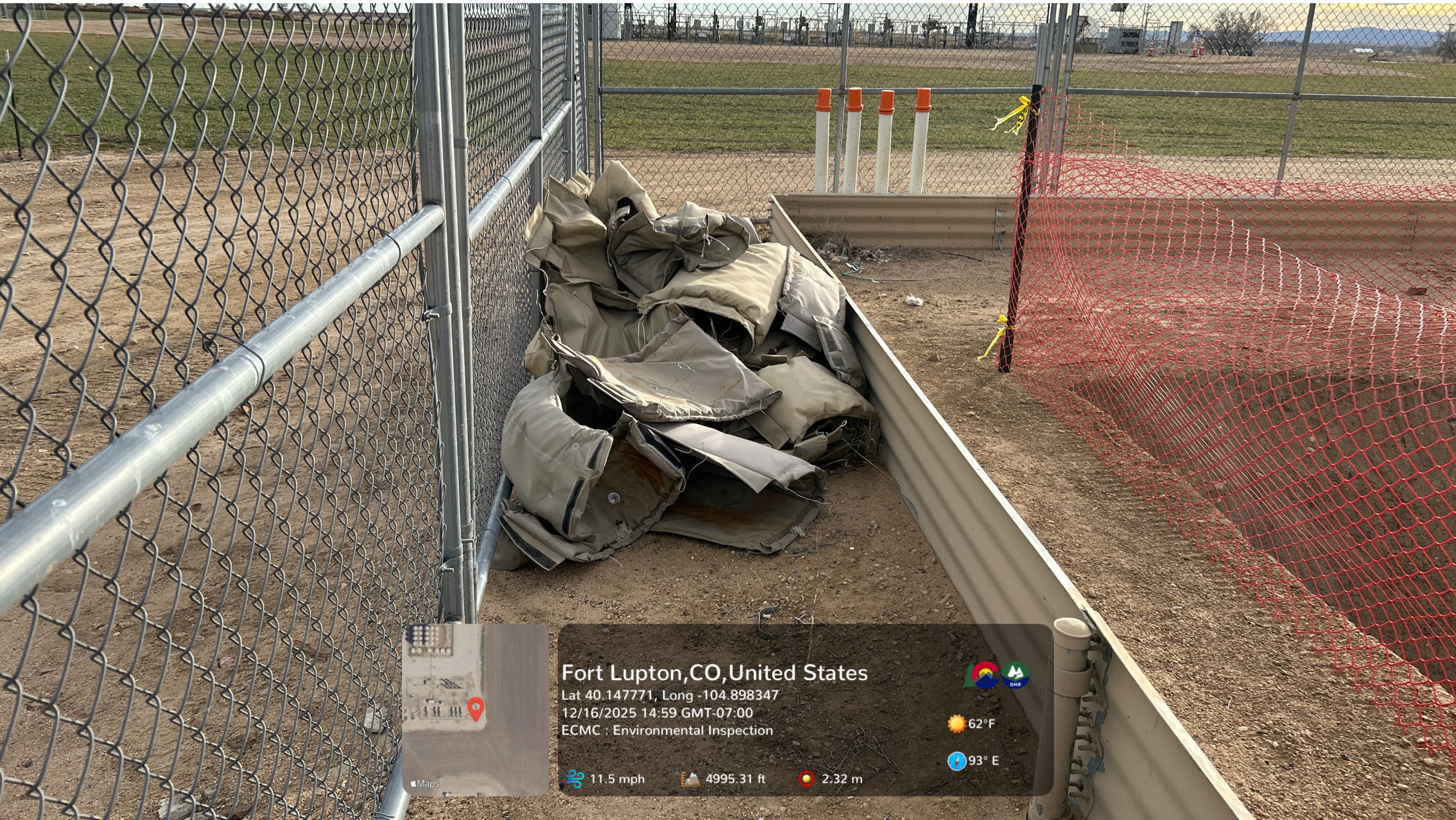
Pipe insulation is visible next to the spill location.
