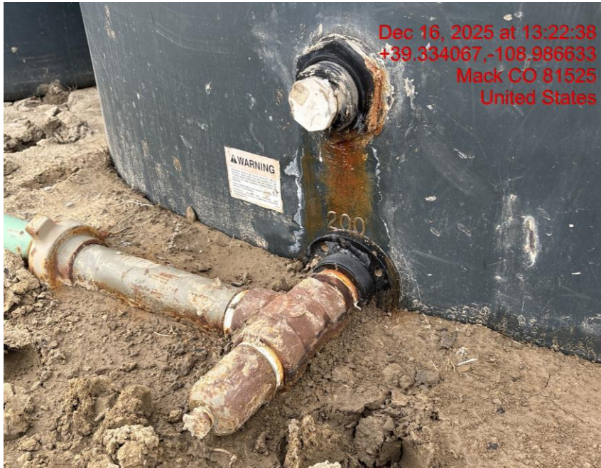
Leak on Tank Plug – Photo #02043
