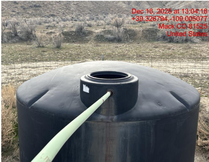
Missing Tank Cover/Wildlife Entry Hazard – Photo #02033
