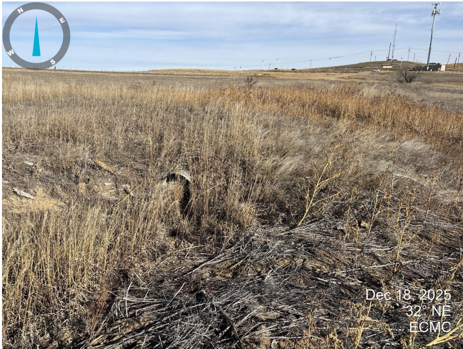
Photo 3. Picture taken near the location looking east across the access road. A culvert remains in place under the access road.
