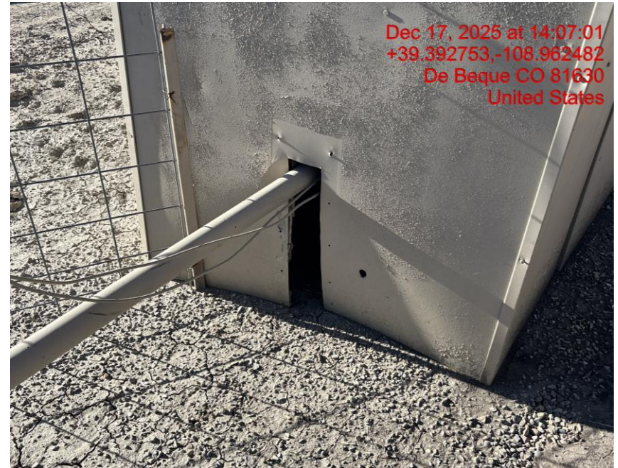
Wildlife Entry Hazard – Photo #02103
