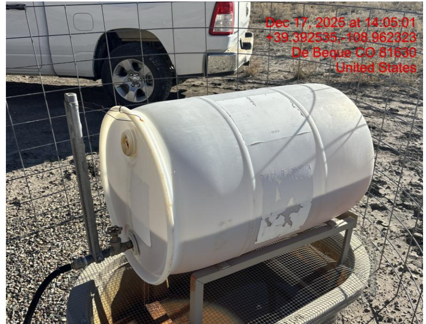
Unlabeled Chemical Tank (Fluid in Tank) – Photo #02096
