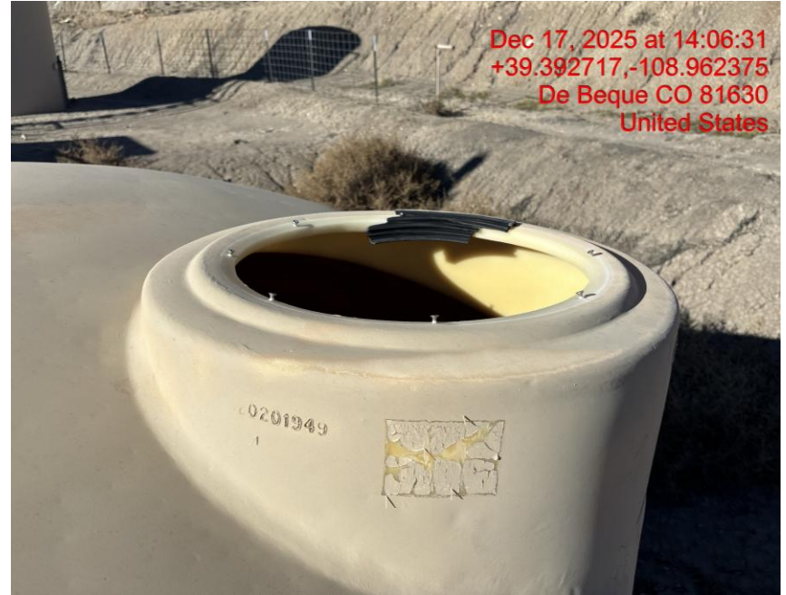
Missing Cover/Wildlife Entry Hazard on Plastic AST – Photo #02100
