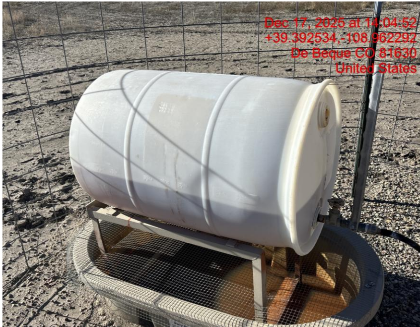
Unlabeled Chemical Tank (Fluid in Tank) – Photo #02095
