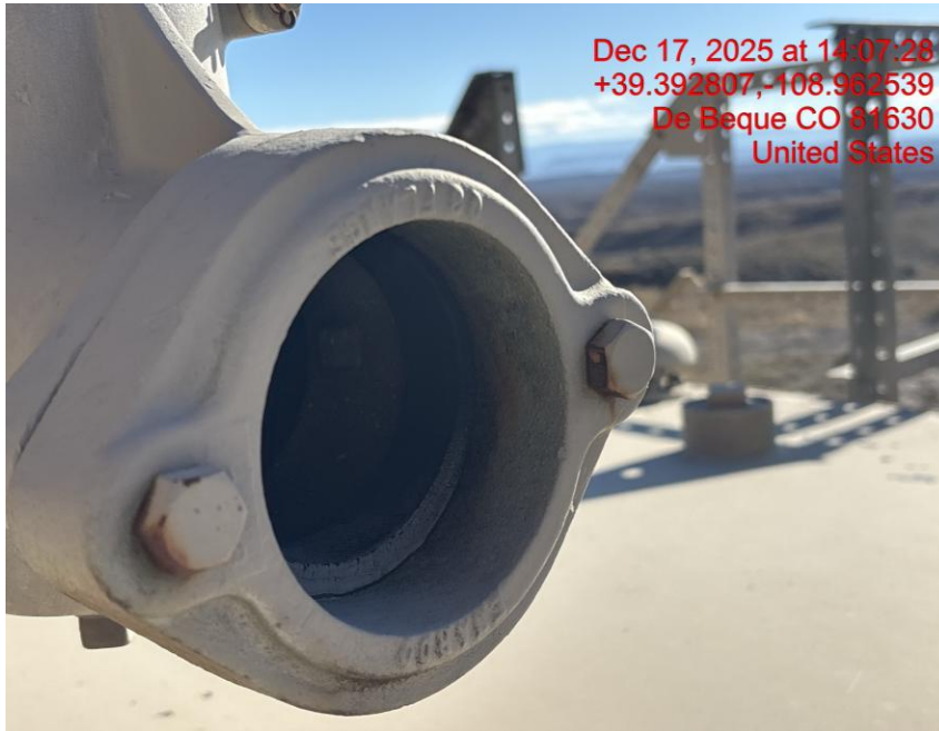
Open-Ended Line on Steel AST – Photo #02105
