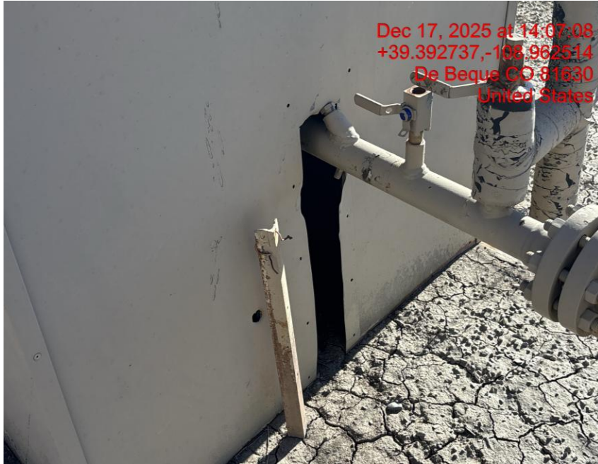
Wildlife Entry Hazard – Photo #02104
