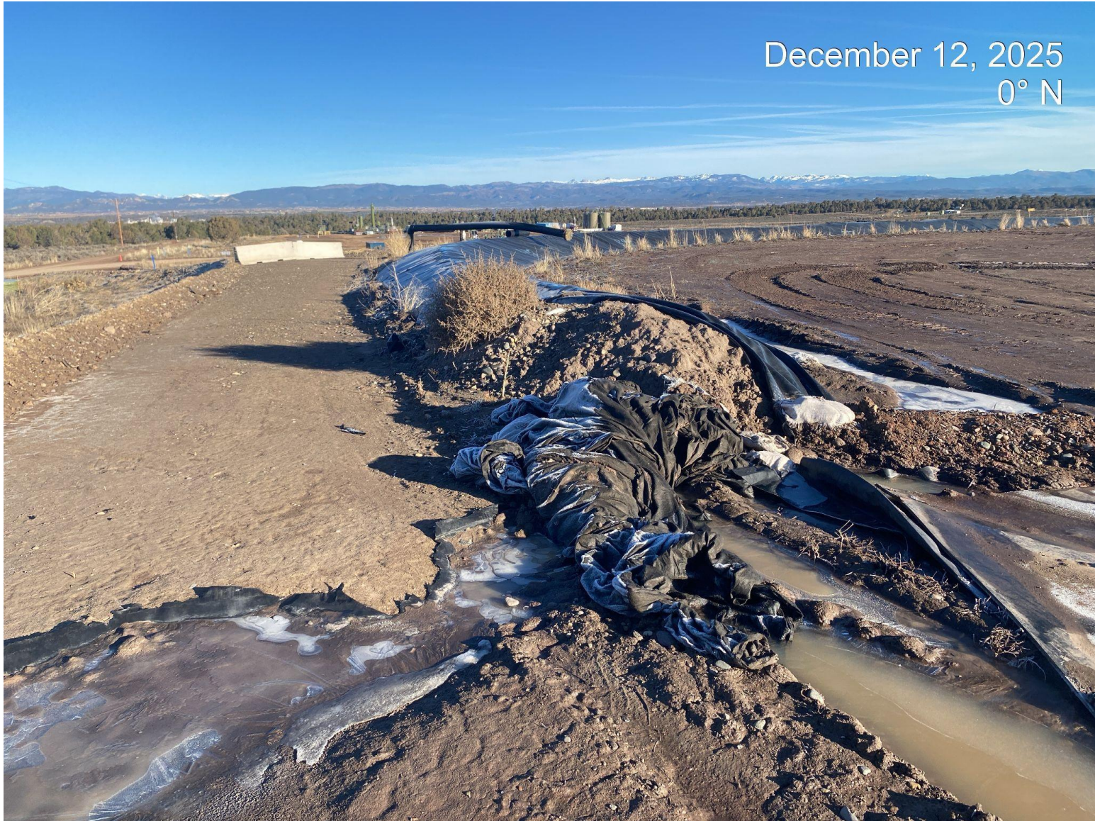
Photo 2. Unused fabric/mats piled on the western edge of the TUA pad.
