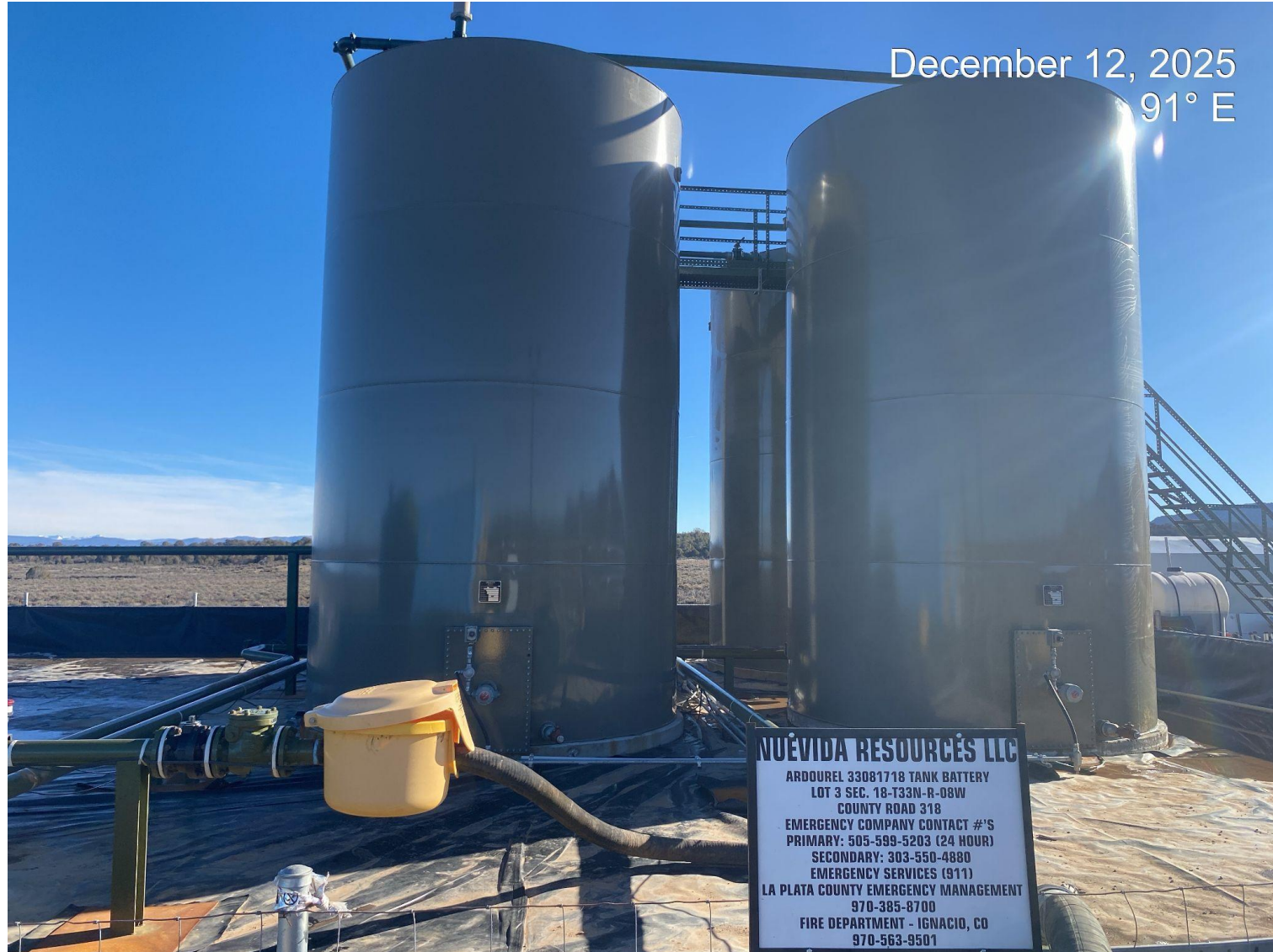
Photo 12. Tanks in the northeast corner of the well pad remain unmarked. Physical markings on each individual tank is required.
