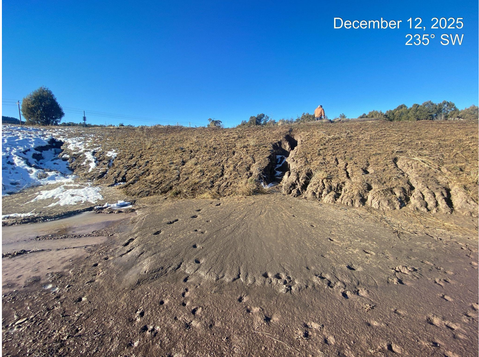
Photo 3. Gully erosion (and sediment deposition) persisting in the SW corner of the TUA cut slope area.
