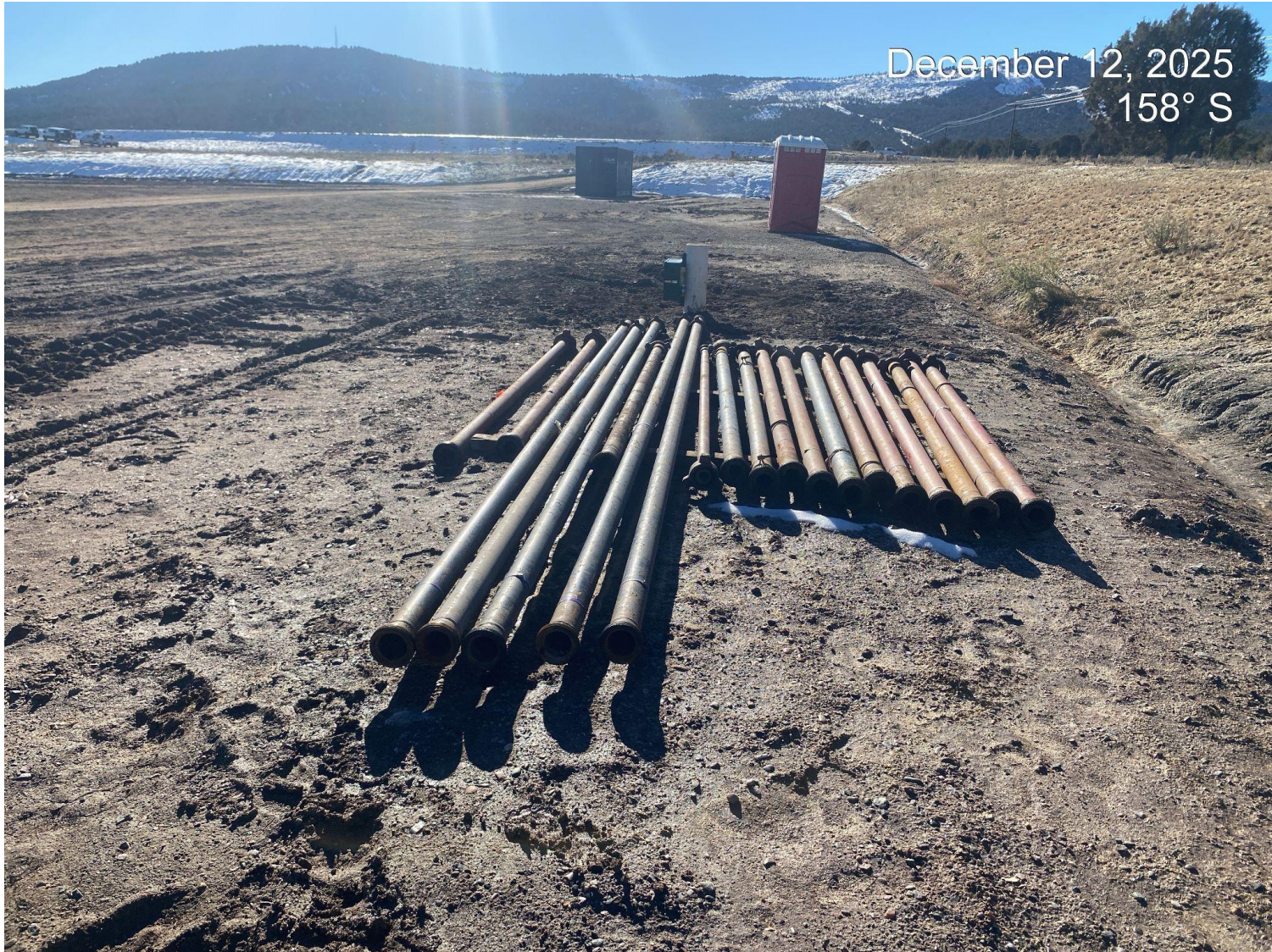
Photo 9. Unused piping stored on the western edge of the well pad.
