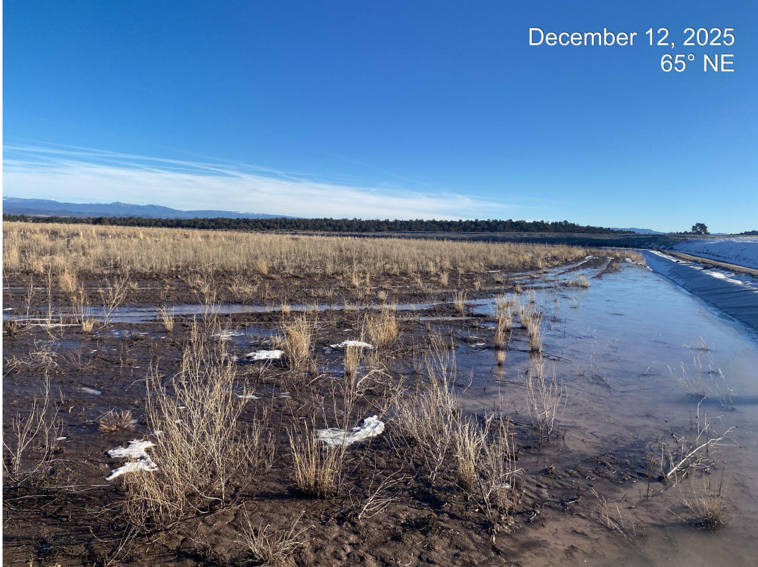
Photo 4. Pooling water observed on the southern edge of the TUA pad.
