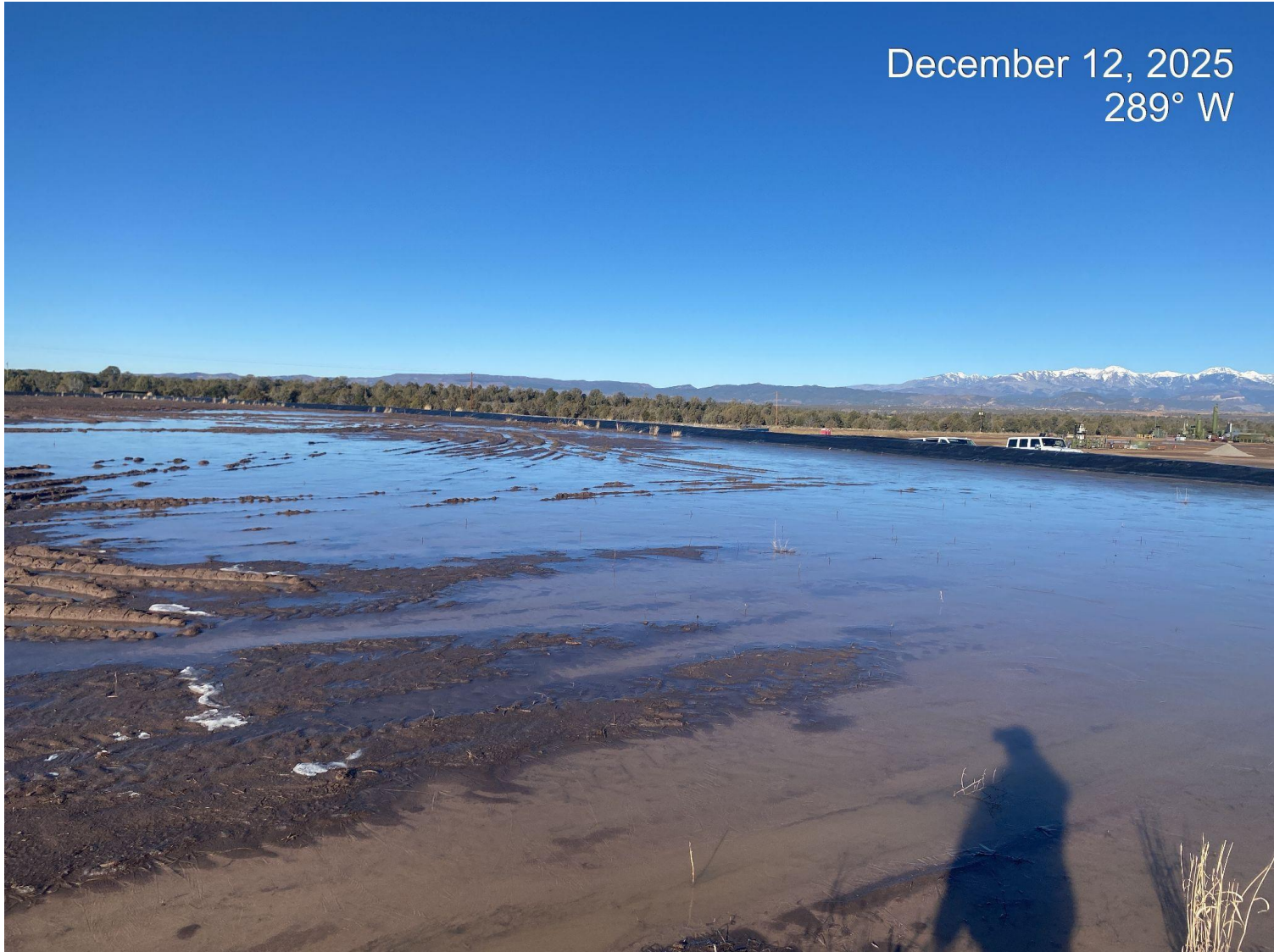
Photo 5. Pooling water occurring in the NE corner and along the northern edge of the TUA pad.
