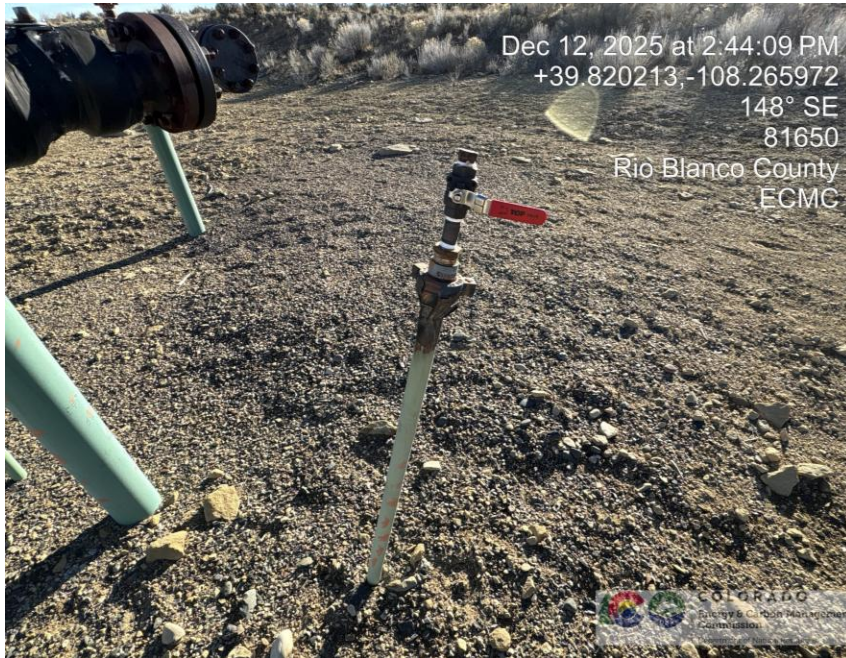
Photo # 0057 Unused flowline lacks lockout tagout (OOSLAT)
