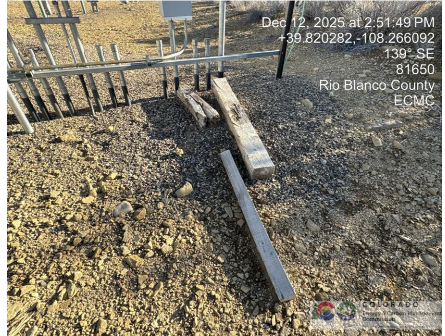
Photo # 0069 Debris on location
