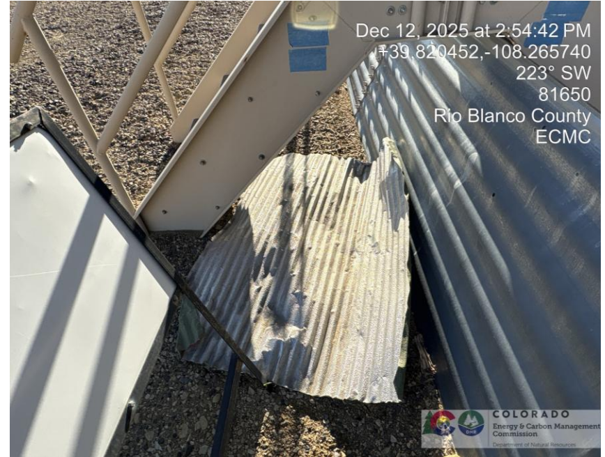
Photo # 0073 Debris on location
