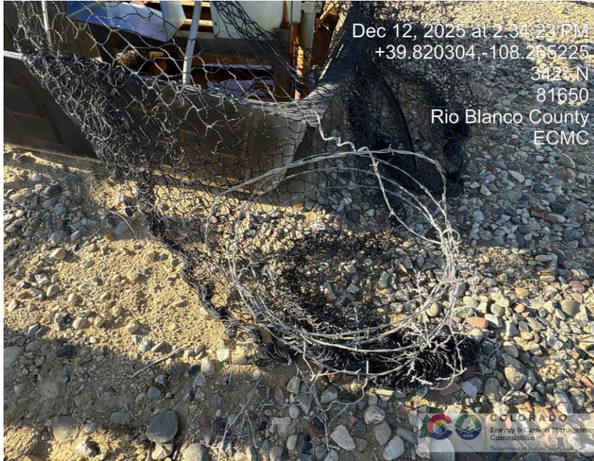
Photo # 0034 Debris on location
