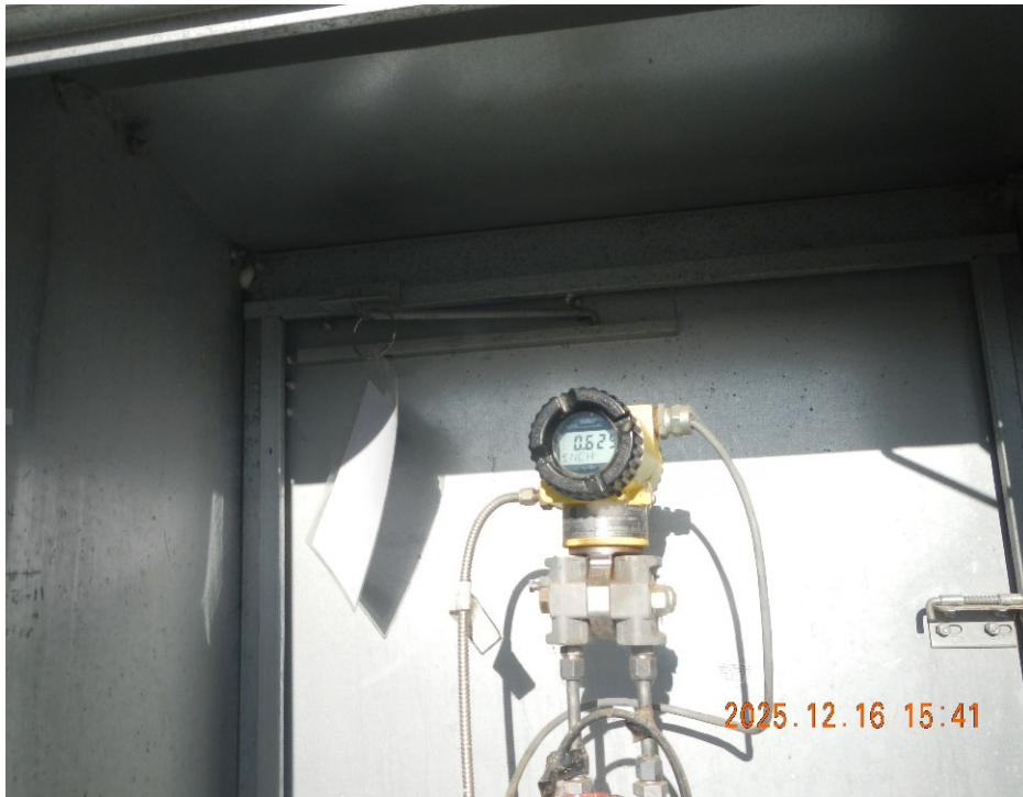
3. Gas Meter inside Flowline mounted Meter Box.
