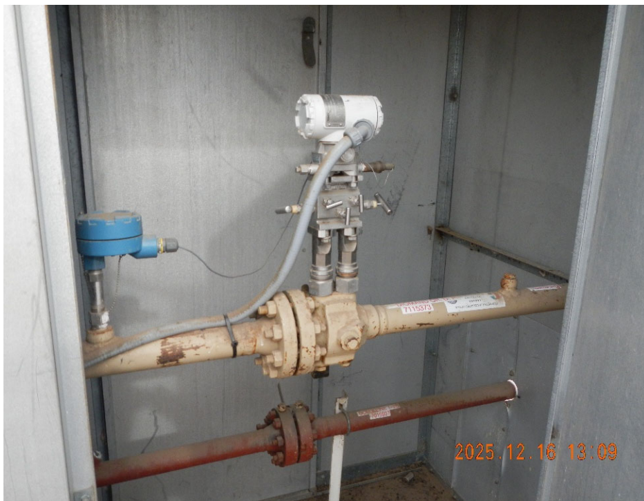
6. Gas meter inside meter shed.
