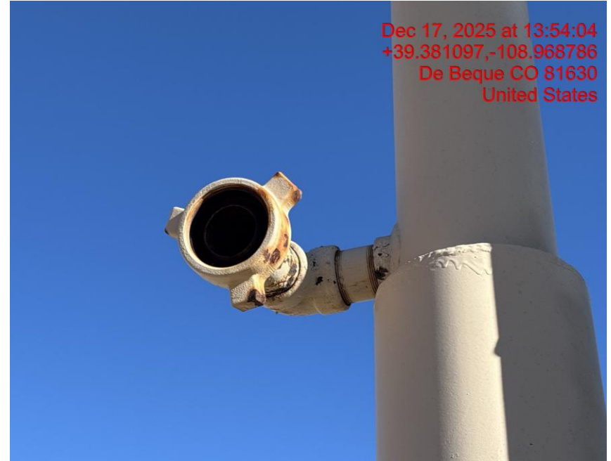
Open-Ended Line – Photo #02091
