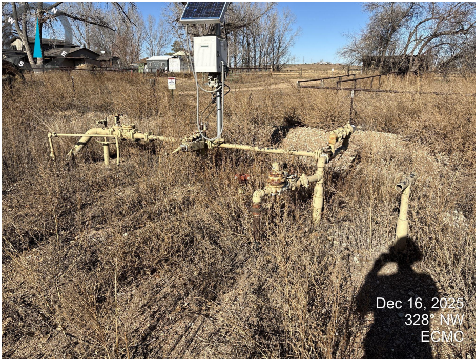
Photo 3. Weeds in contact with equipment.
