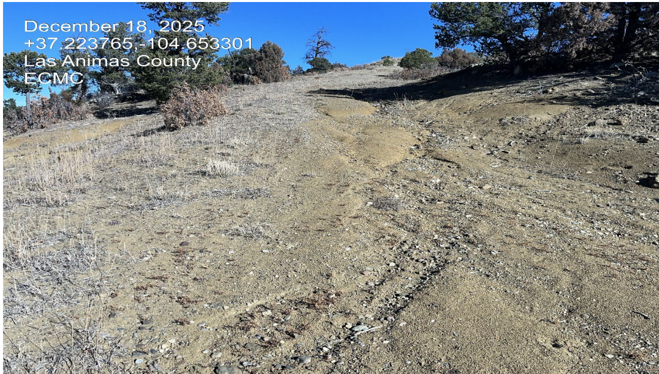
Photo 1. Facing northeast toward the access road. There are signs of erosion in this area which is not stabilized.
