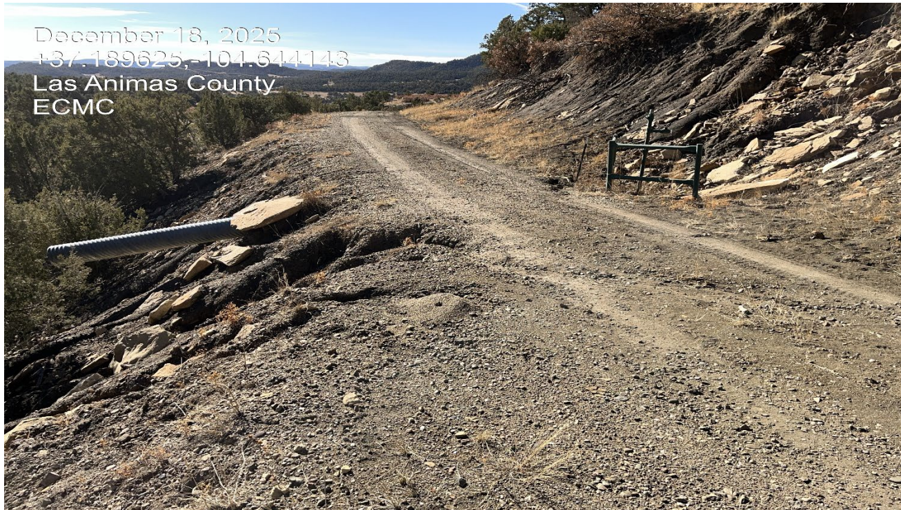
Photo 1. Facing southeast along the access road. There is erosion along the side of the road and stormwater is not being directed toward the culvert.
