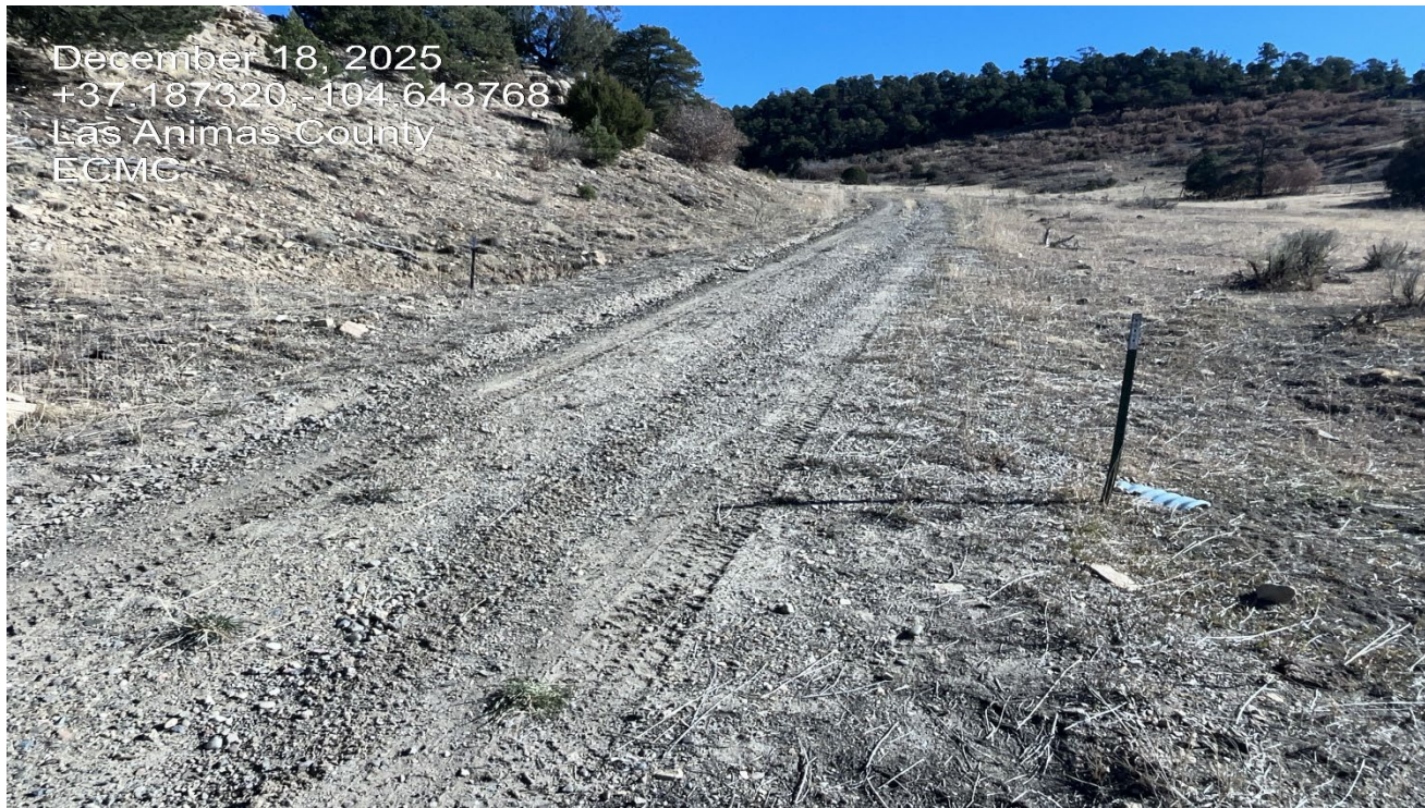
Photo 2. Facing east along the access road. This culvert is filled in with sediment..
