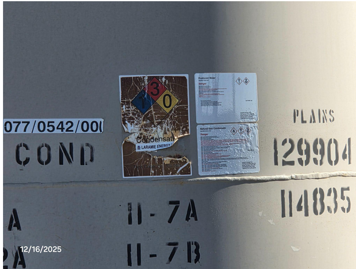
Photo 3: Photo shows Label on tank is peeling. Maintenance advised.
