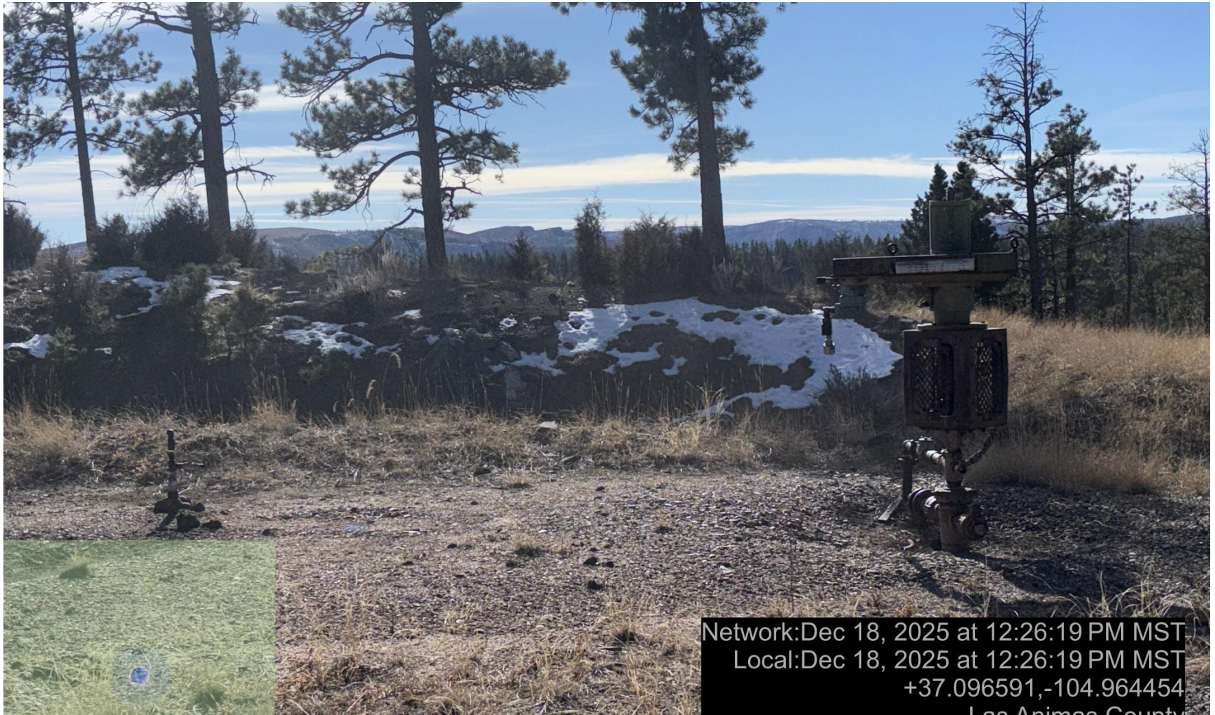
PHOTO 3: UNUSED EQUIPMENT (1" RISER). REMOVE OR MARK RISER PER RULE 606. CA DATE 1-18-2026.
