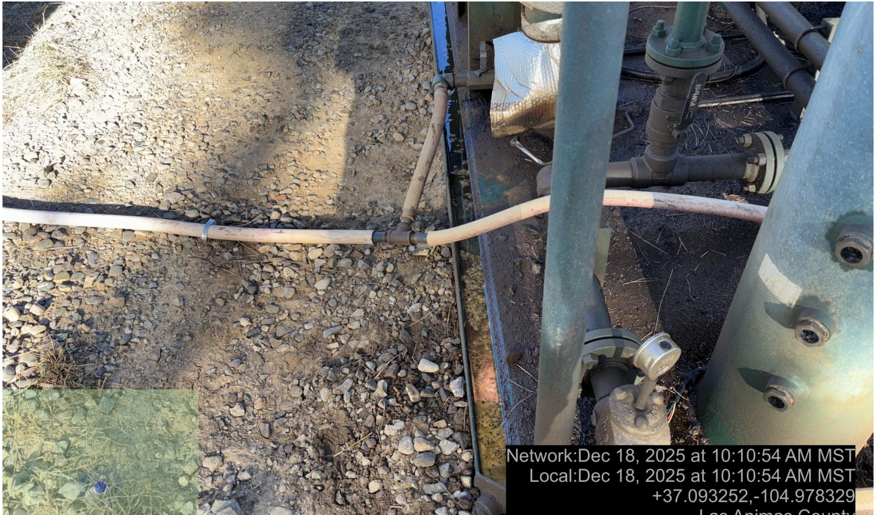
PHOTO 5: AREA OF IMPACTED SOIL NEAR COMPRESSOR. Conduct maintenance on equipment, cleanup stained material and review self inspection processes. COMPLY WITH RULE 1002,,(2).D. CA DATE 1-18-2025.
