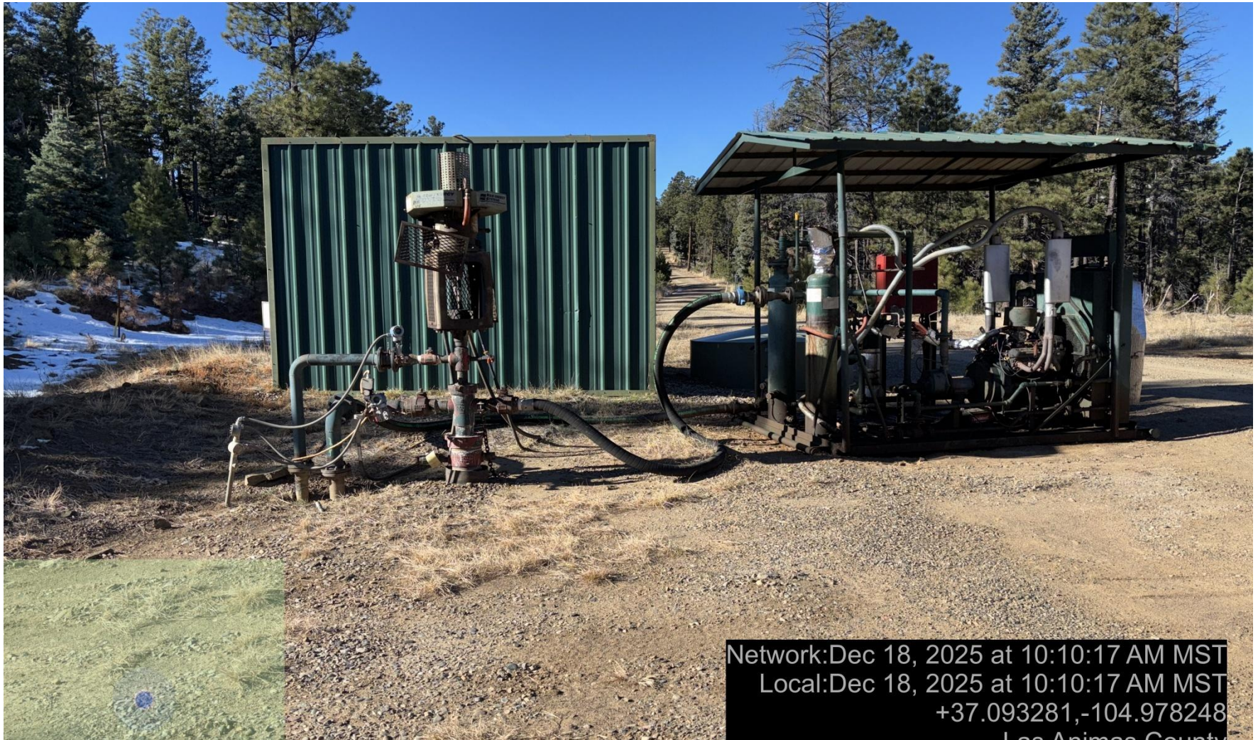
PHOTO 3: WELLHEAD AND EQUIPMENT.
