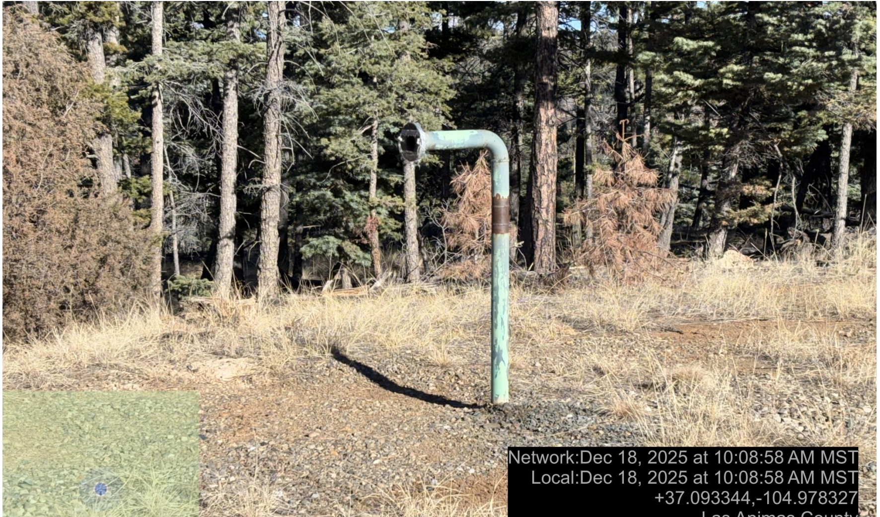
PHOTO 4: UNUSED OR UNUSEFUL EQUIPMENT (3" RISER OPEN TO ATMOSPHERE ON NORTH SIDE OF LOCATION). REMOVE UNUSED OR UNUSEFUL EQUIPMENT PER RULE 606. CA DATE 1-18-2025.
