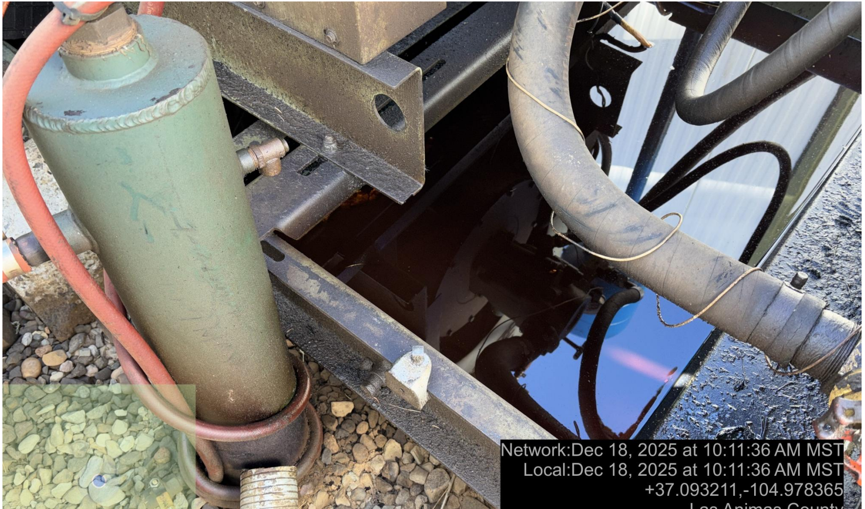
PHOTO 6: OIL IN PRIME MOVER ENGINE SKID WITHOUT WILDLIFE PROTECTION NET OR SCREEN (IT APPEARS THE ENGINE OIL HAS BEEN DRAINED DIRECTLY INTO ENGINE SKID AND LEFT, THIS PRACTICE SHOULD STOP IMMEDIATELY). DRAIN OILY WASTE REPAIR ALL LEAKS AND REMOVE IMPACTED SOIL PER RULE 1002..(2).D & 1002.f.(2)B, Comply with general provisions of the oil and gas act for wildlife protection AND SB-181. CA DATE 12-19-2025.
