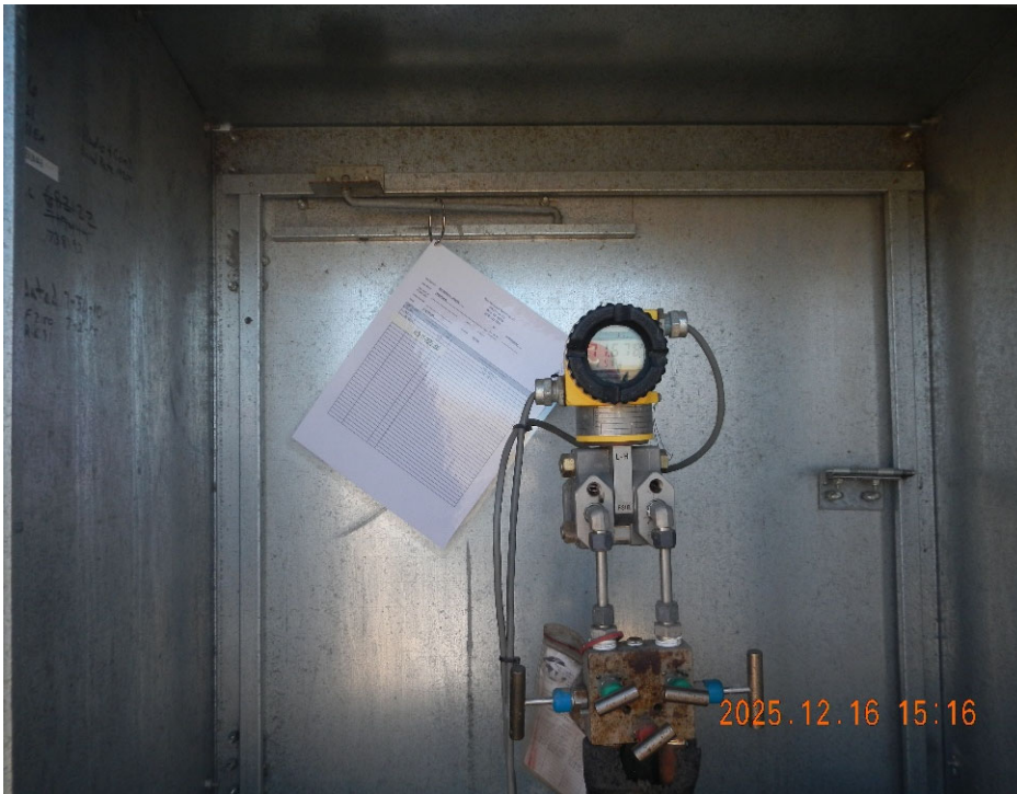
3. Gas Meter inside Flowline mounted Meter Box.
