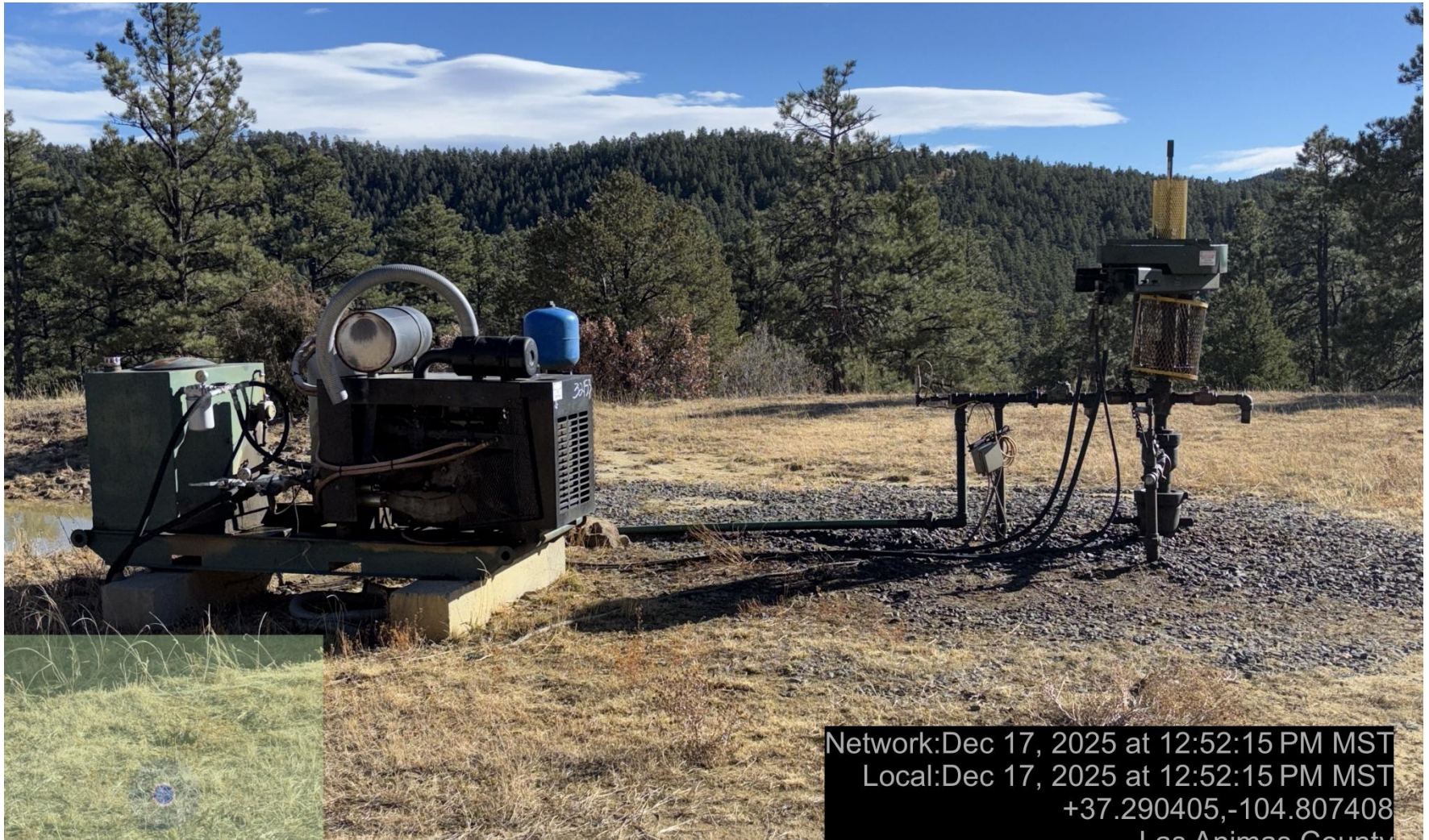
PHOTO 4: ORIG. WELLHEAD AND EQUIPMENT.
