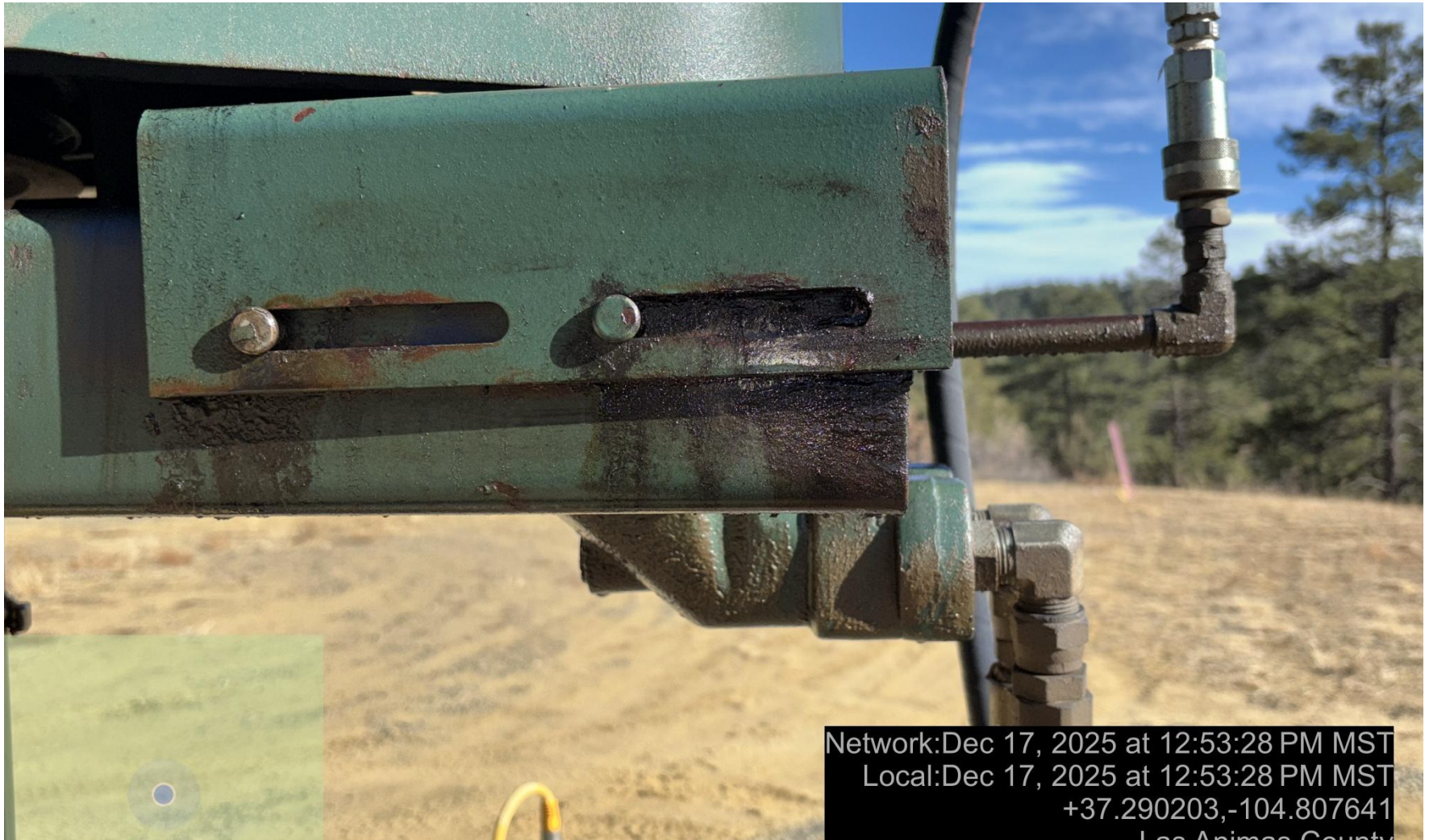
PHOTO 7: DIRVEHEAD ON TR WELL IS LEAKING HYDRAULIC FLUID. Securely fasten all valves, pipes, fittings, and Production Facilities to ensure good mechanical condition, inspect at regular intervals and maintain in good mechanical condition. Engineer, operate, and maintain equipment within the manufacturer's recommended specifications per Rule 608.e. CA DATE 12-22-2025.
