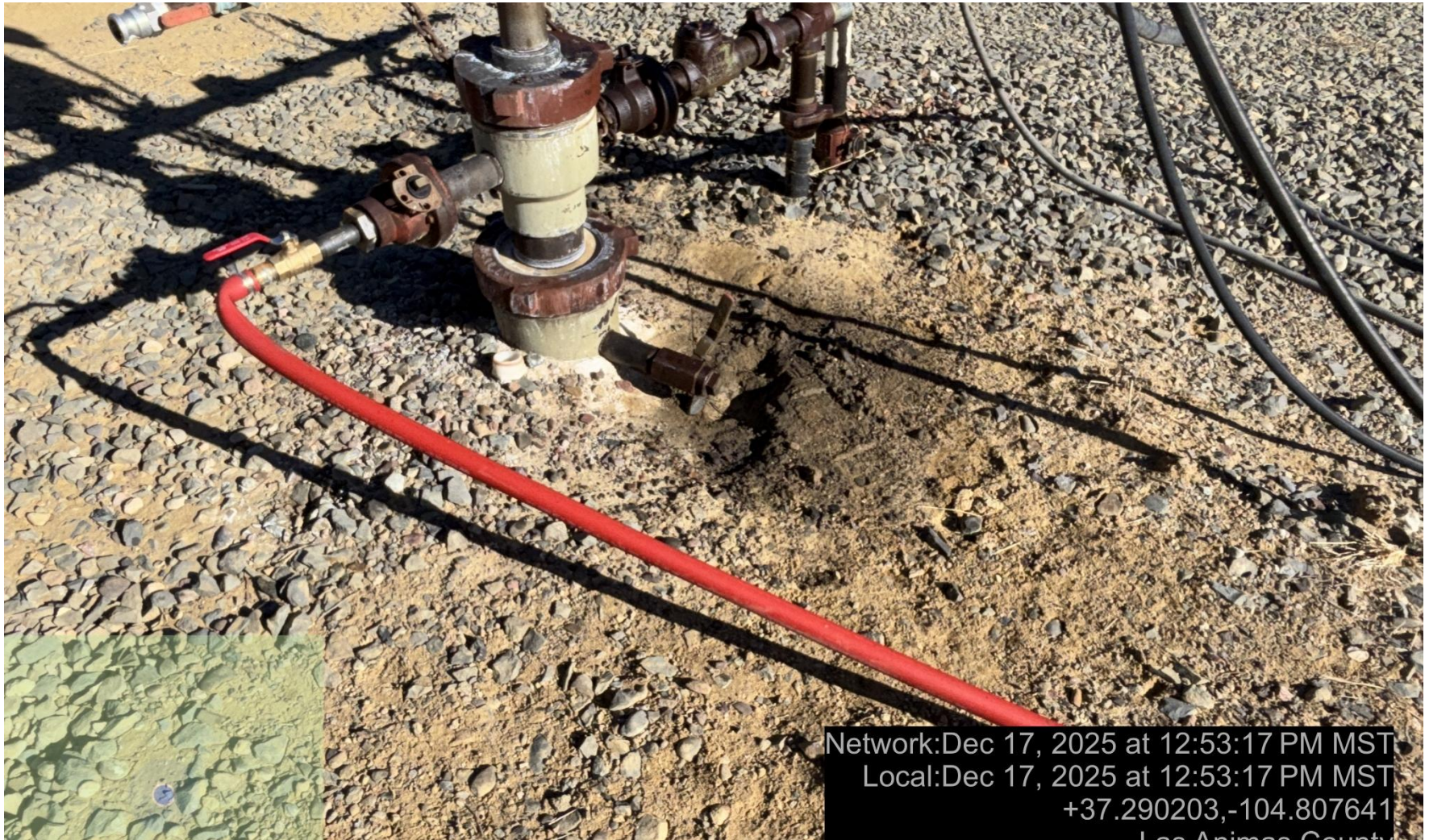
PHOTO 6: AREA OF IMPACTED SOIL AROUND TR WELLHEAD. Conduct maintenance on equipment, cleanup stained material and review self inspection processes. COMPLY WITH RULE 1002,.(2).D. CA DATE 1/1/2026.
