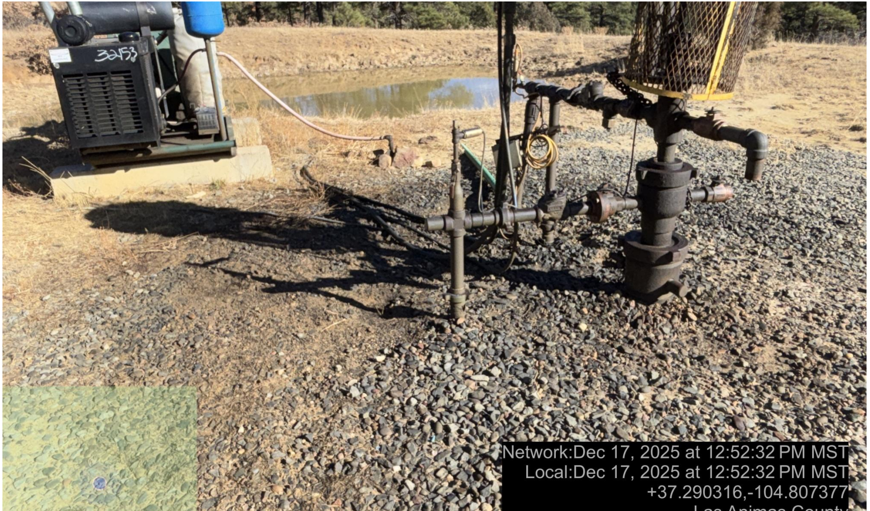
PHOTO 5: AREA OF IMPACTED SOIL AROUND ORIGINAL WELL WELLHEAD. Conduct maintenance on equipment, cleanup stained material and review self inspection processes. COMPLY WITH RULE 1002,.(2).D. CA DATE 1/1/2026.
