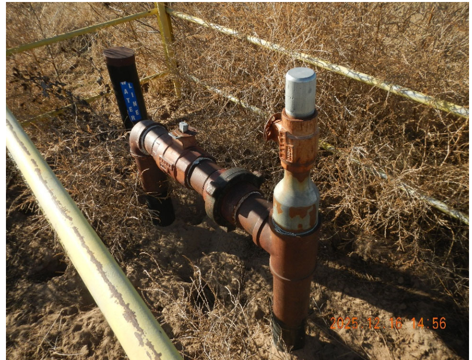
4. Flowline and water valves access at well location.
