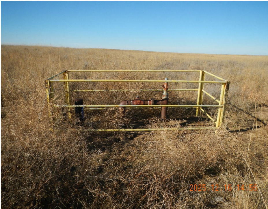
5. View of flowline riser and water valves with welded tube barrier at well location.
