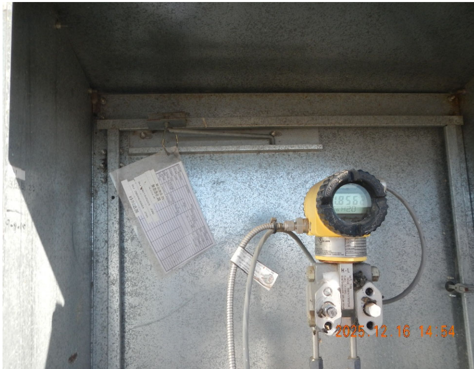
3. Gas Meter inside Flowline mounted Meter Box.
