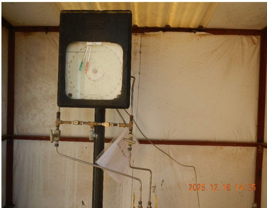
5. Gas Meter inside Meter Shed.
