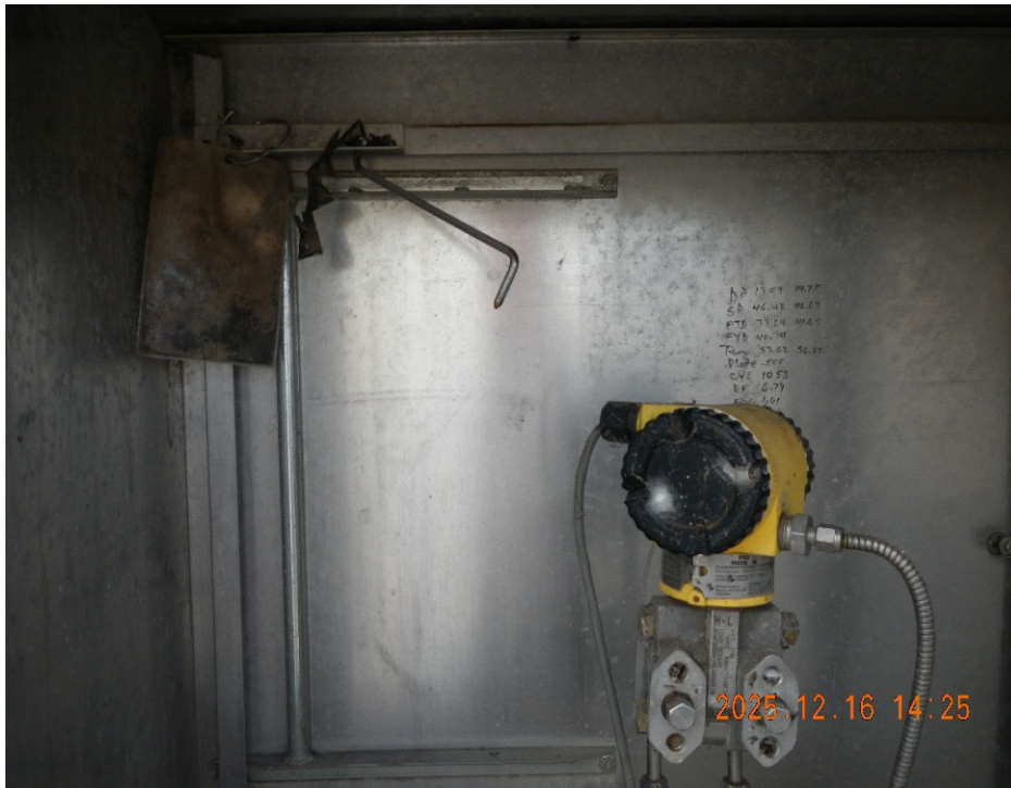
3. Gas Meter inside Flowline mounted Meter Box.
