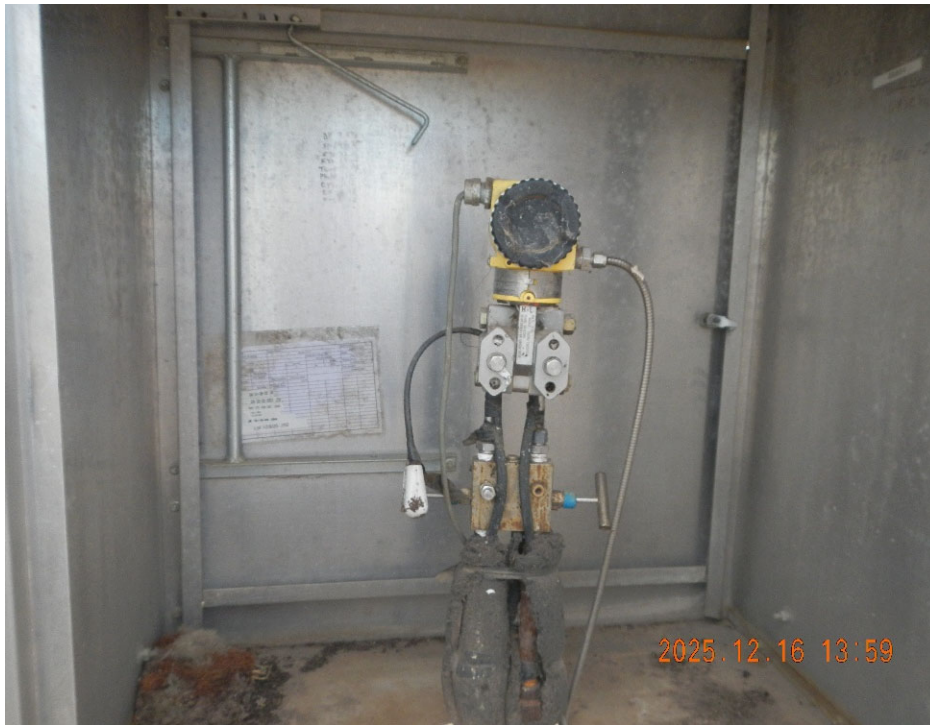
3. Gas Meter inside Flowline mounted Meter Box.
