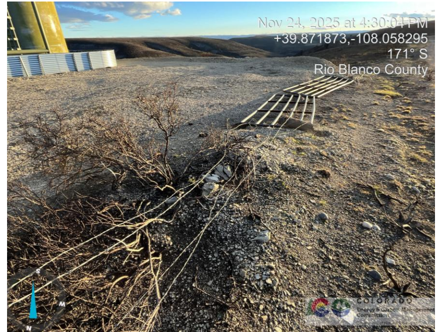
Photo # 4563 Loose barbed wire fencing on location/wildlife hazard & fencing is in disrepair
