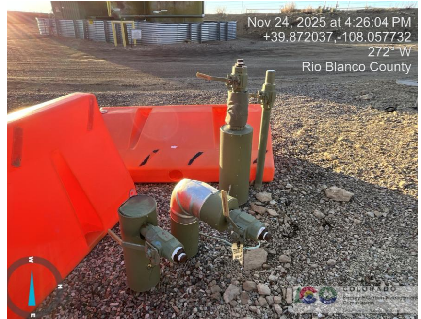
Photo # 4558 Unused flowlines lack lockout tagout (OOSLAT)
