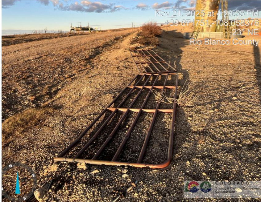
Photo # 4560 Loose barbed wire fencing on location/wildlife hazard & fencing is in disrepair
