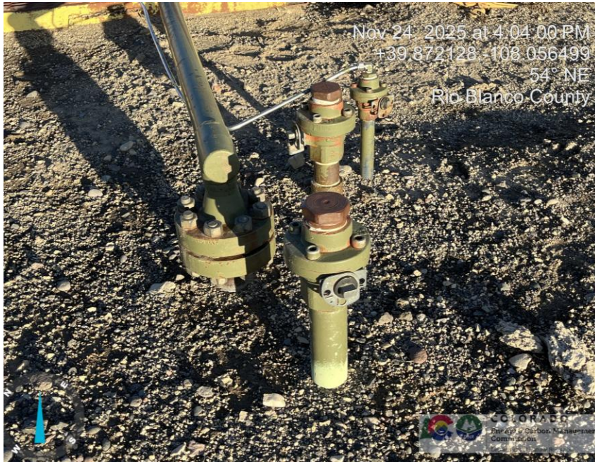
Photo # 4525 Unused flowlines lack lockout tagout (OOSLAT)
