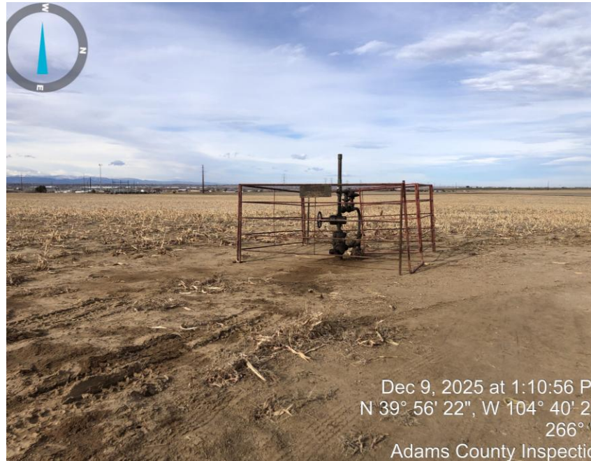
Photo #3 Well head.
