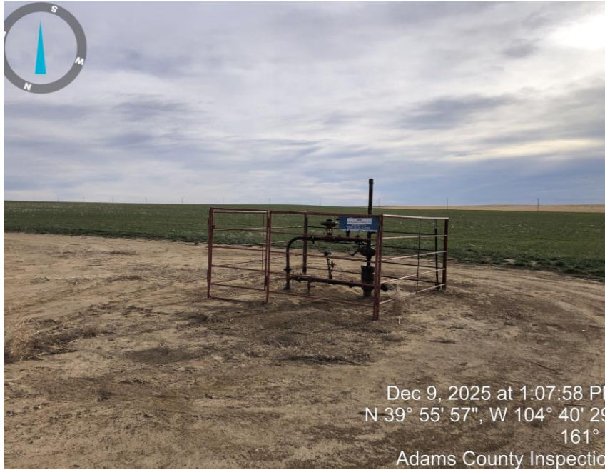
Photo #3 Well head.
