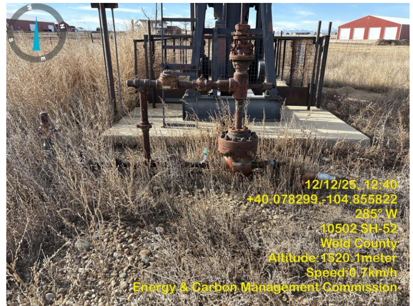
Photo 4 Tall dead vegetation around the wellhead .
