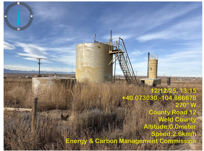
Photo 2 Tank battery overrun with dead vegetation.
