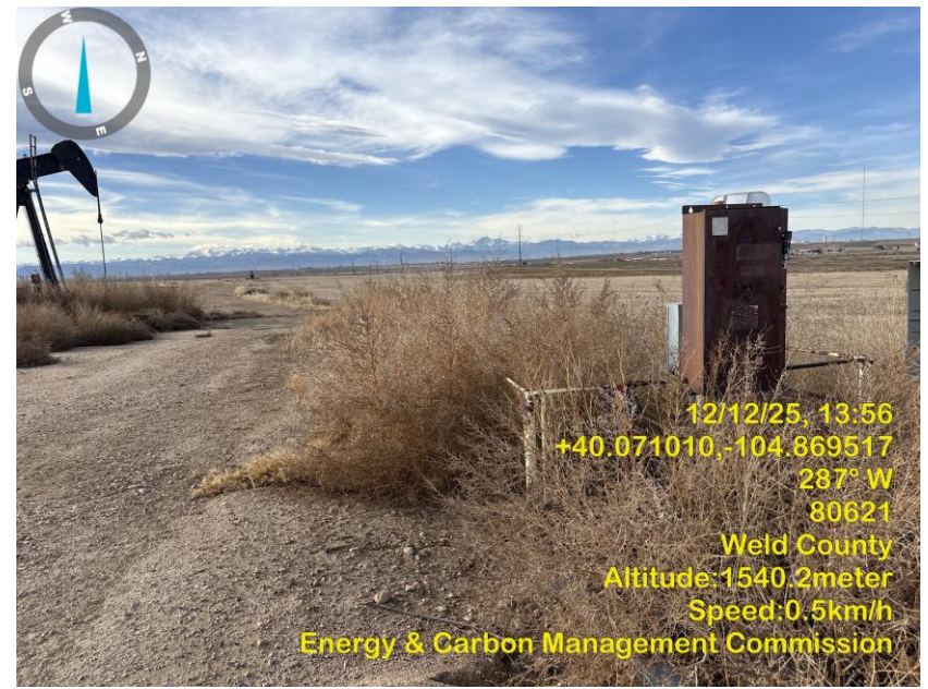
Photo 2 Ancillary equipment overrun with dead vegetation.
