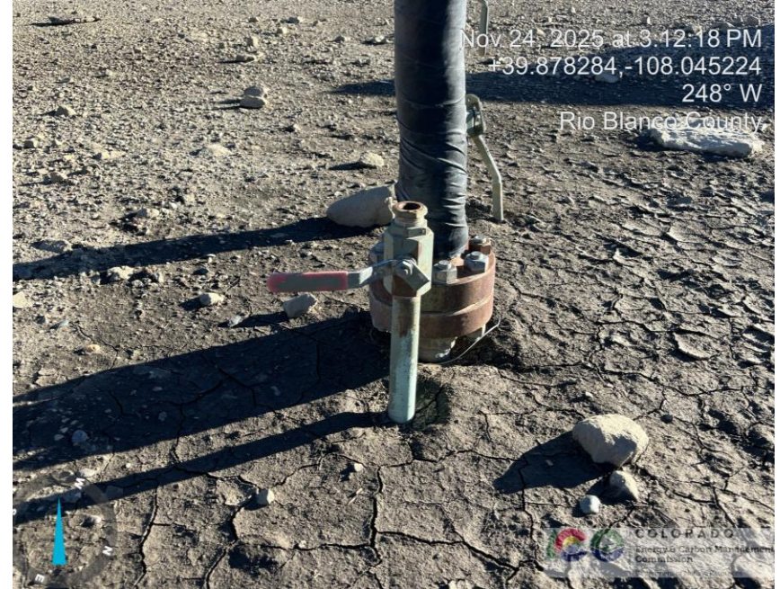
Photo # 4493 Unused flowline lack lockout tagout (OOSLAT
