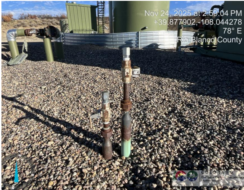
Photo # 4487 Unused flowlines lack lockout tagout (OOSLAT)
