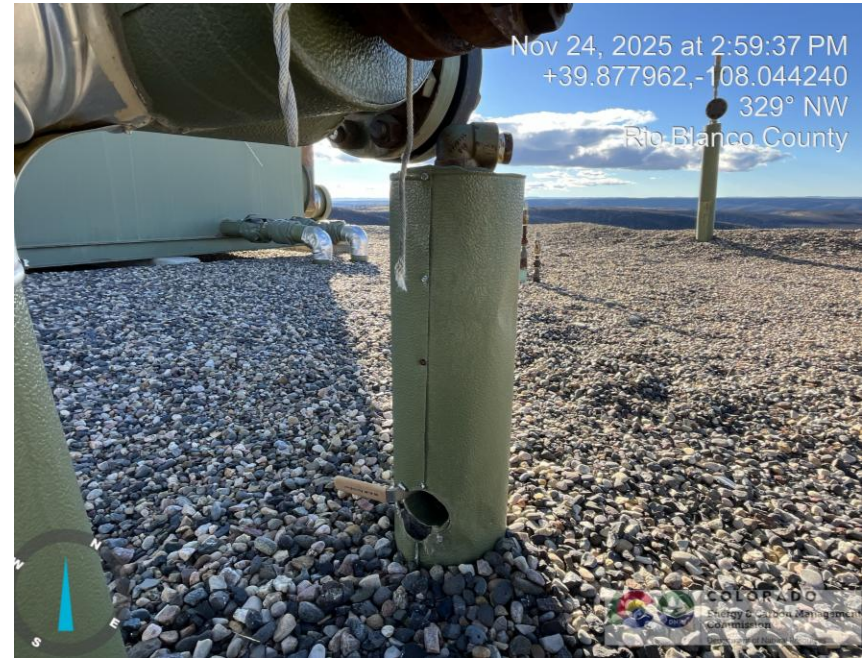
Photo # 4488 Unused flowline lack lockout tagout (OOSLAT)
