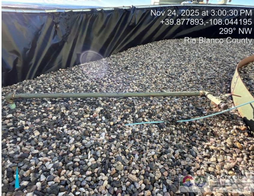
Photo # 4489 Unused flowline lack lockout tagout (OOSLAT
