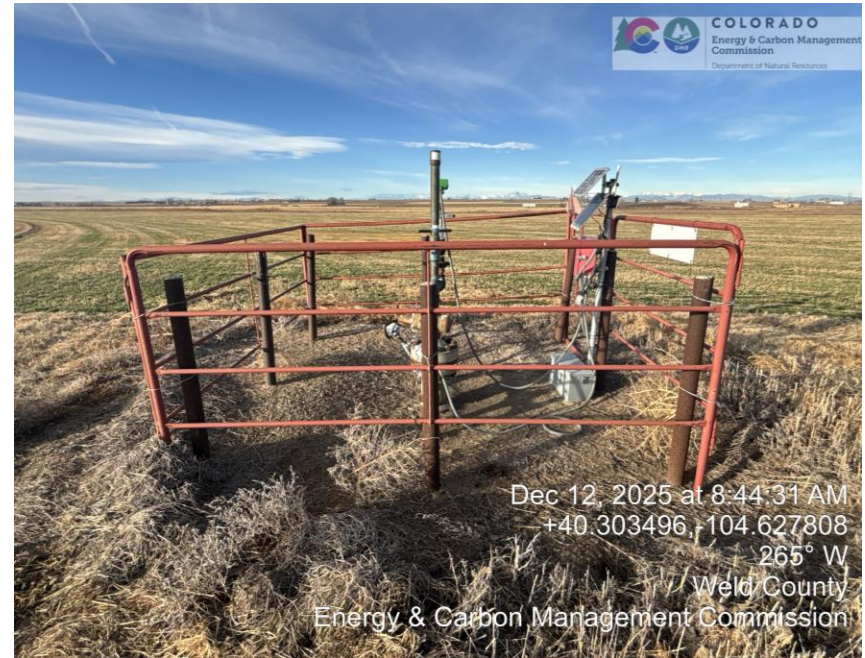
Photo 2 well head and equipment
