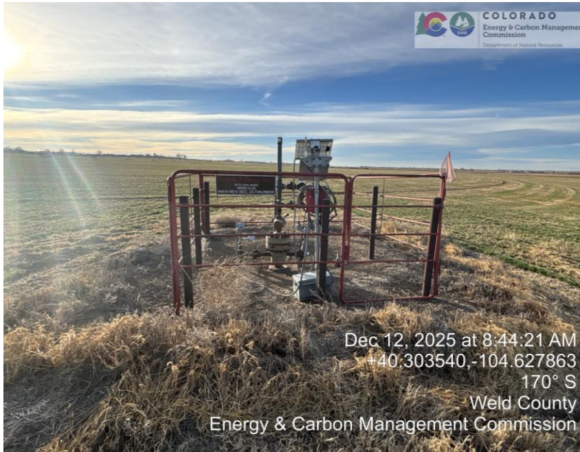
Photo 1 well head and equipment
