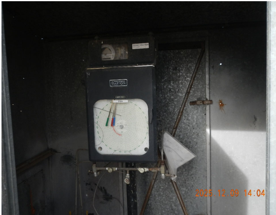
3. Gas Meter inside Meter Shed.
