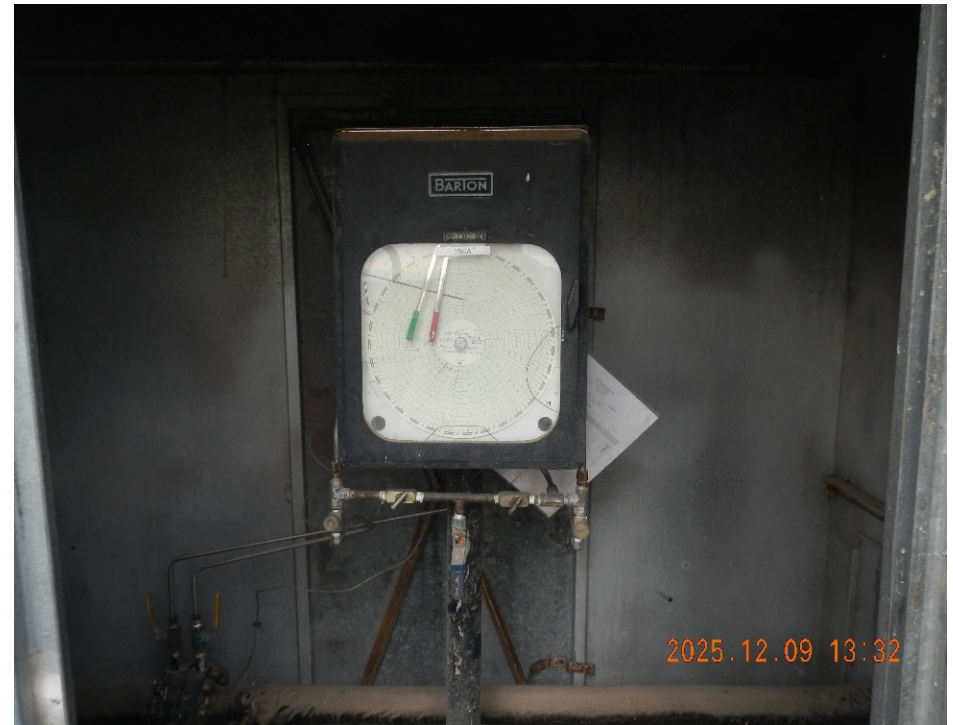
4. Gas Meter inside Meter Shed.
