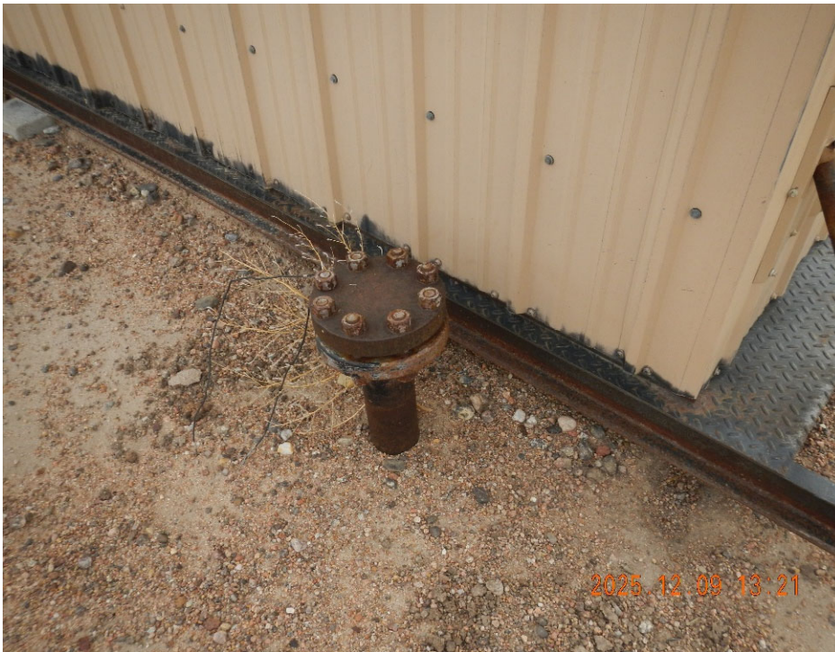
7. Flowline riser at gathering location with bolted cap.
