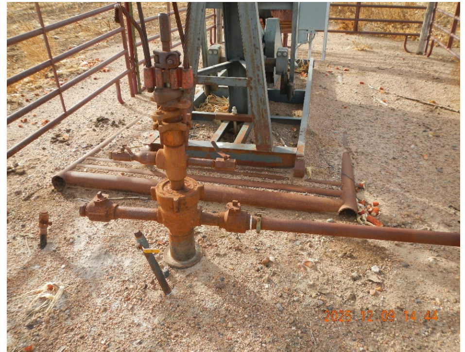
2. View of wellhead. Note open-ended line on tubing water leg.
