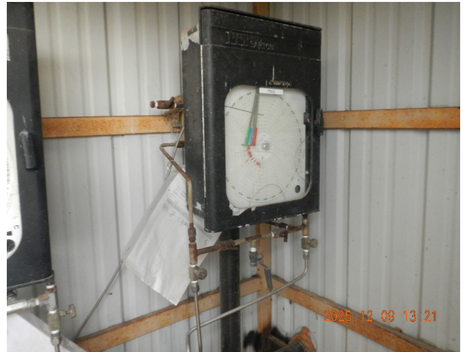
6. Gas meter inside meter shed.
