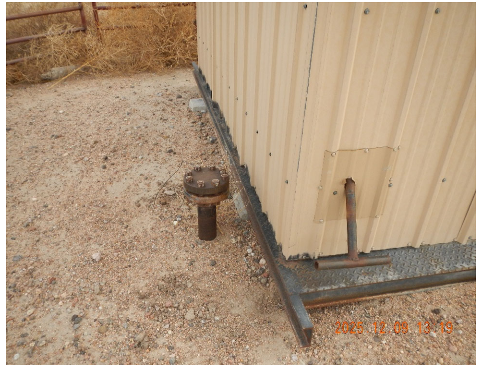
6. Flowline riser with bolted cap at gathering location.
