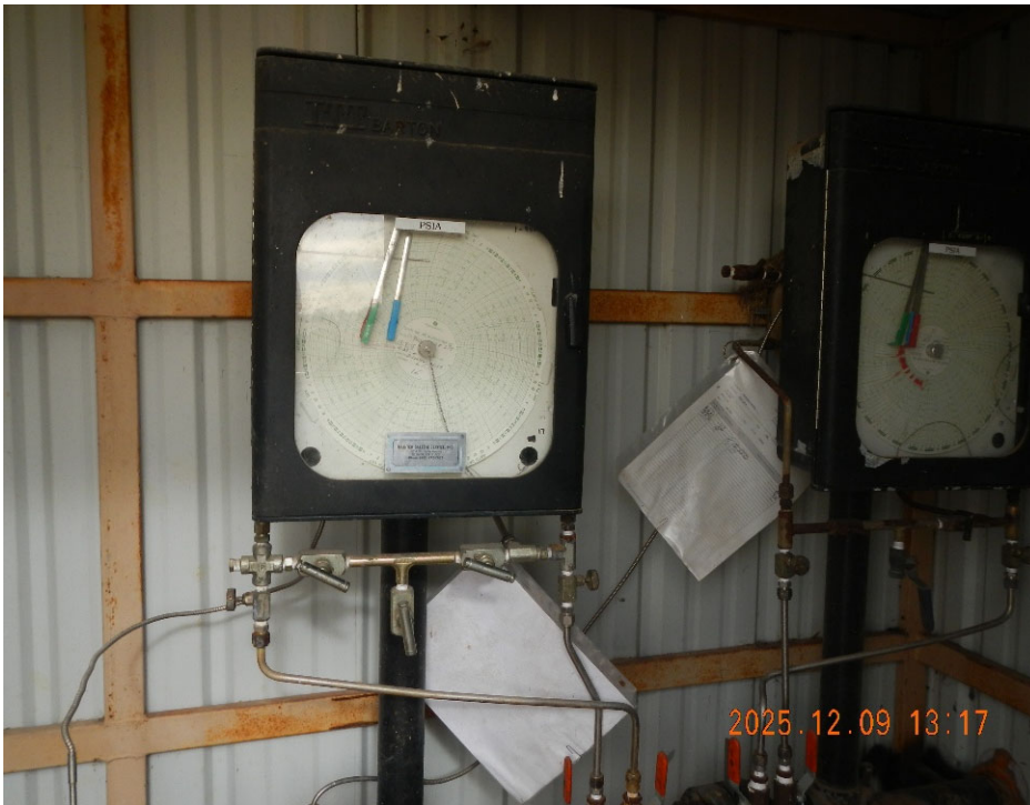
5. Gas Meter inside Meter Shed.
