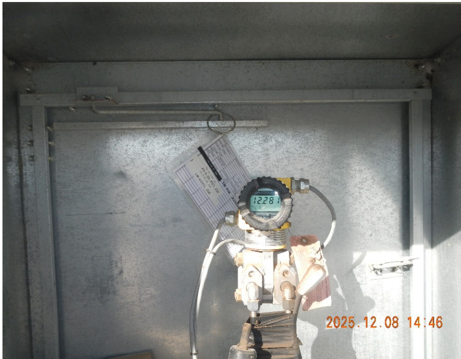
3. Gas Meter inside Meter Box.
