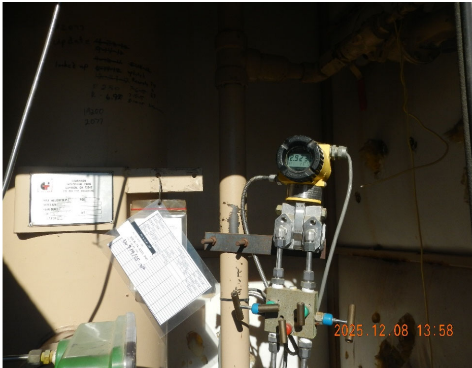
7. Gas Meter inside Meter Shed.
