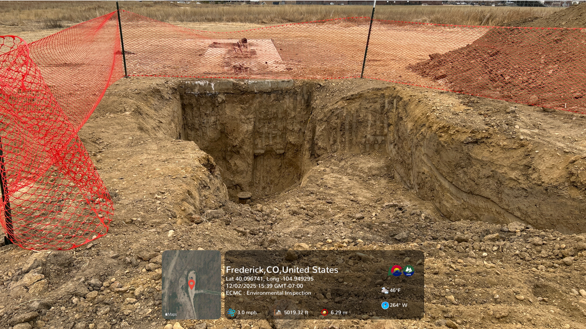
Looking at the open excavation. Orange construction fencing partially surrounds the excavation.
