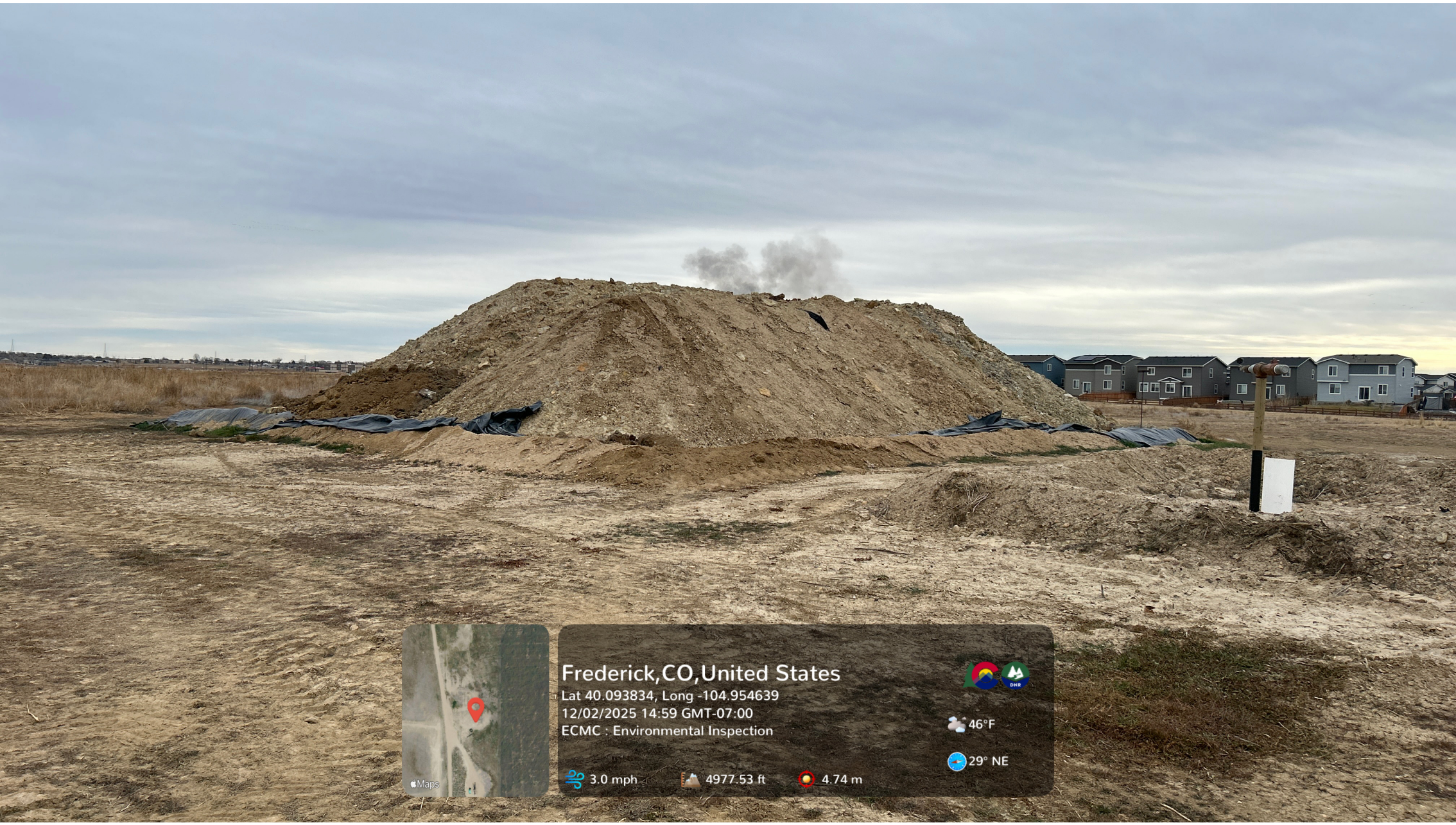
Looking at the east stockpile. A liner is visible; however, the liner is torn, discontinuous, and overtopped by soil.
