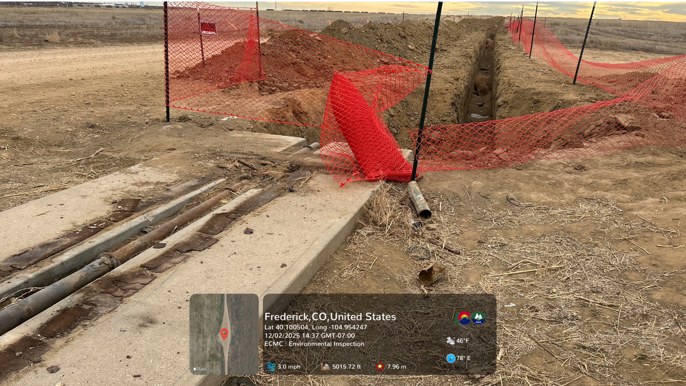
Orange construction fencing partially surrounds an open excavation. Pieces of flowline are visible adjacent to the former well. A trench associated with Flowline Facility ID 478291 is visible running south from the former well.
