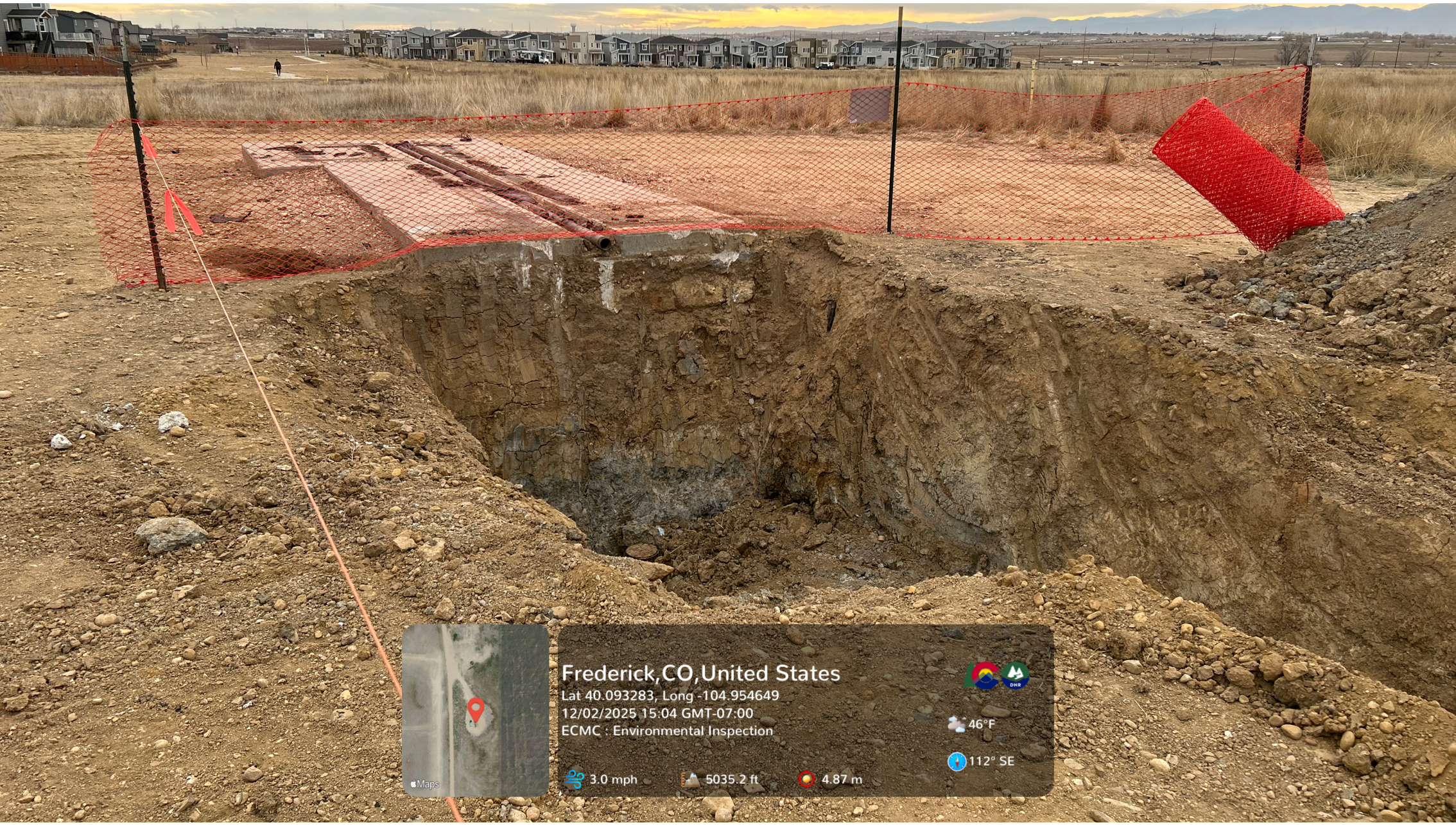
Looking at the former State #3 well. An open excavation is visible. Gray staining is visible in the excavation. Gray staining is visible in the stockpiled soil to the west. A petroleum hydrocarbon odor was observed. The pumping unit has been removed. Multiple residences, a walking path, and a pedestrian are visible in the background.
