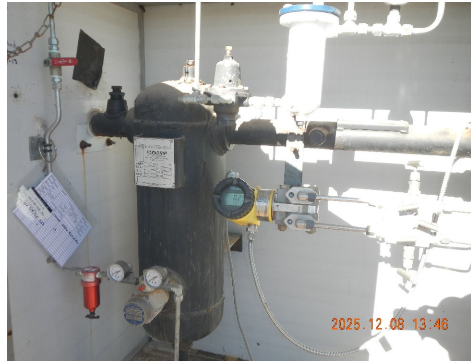
4. View of small vertical separator and gas meter inside Flowline mounted Meter Box.
