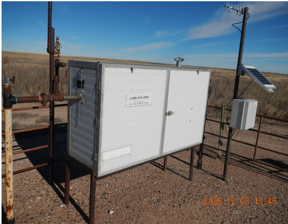
3. View of Flowline mounted Meter Box.
