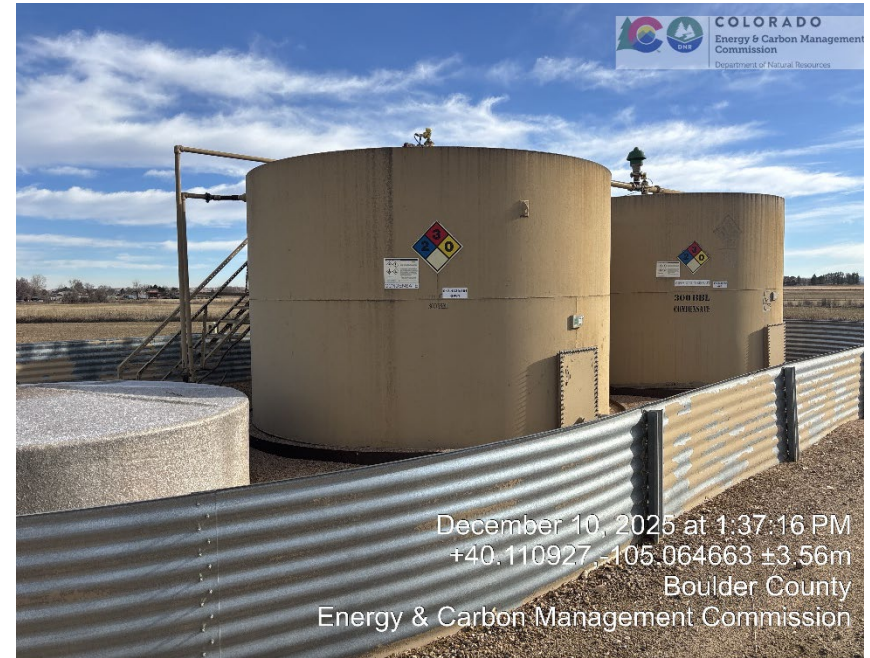
North condensate tank placards
