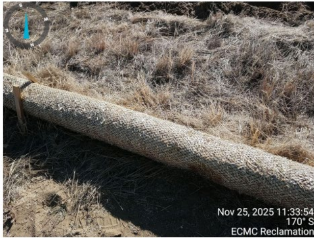
Photo 5. Close up photo taken from a section of the stormwater BMP (straw wattle) illustrating the BMP has not been trenched in per good engineering practices.
