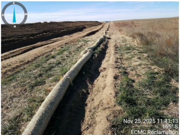
Photo 7. Photo taken from the northern perimeter of location, facing West. Photo illustrates a section of the stormwater BMP (straw wattle) illustrating the BMP has not been trenched in per good engineering practices. It appears that a trench was installed, yet the straw wattle was not placed within the trench. Note- the trench may be too deep for the straw wattle.
