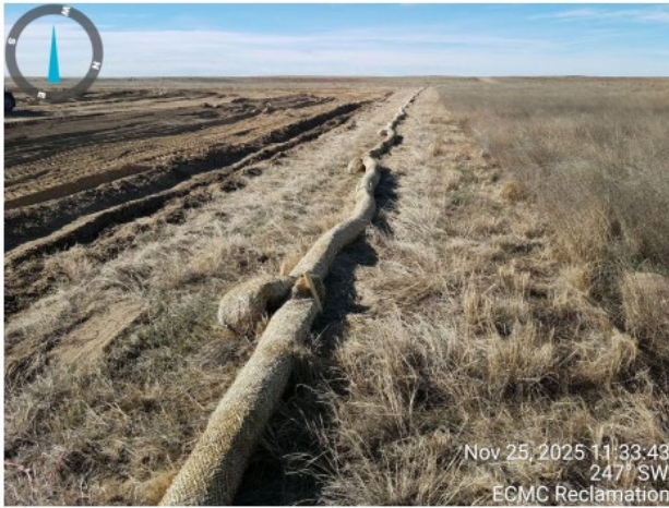
Photo 4. Photo taken from the northwestern perimeter of location, facing West. Photo illustrates the Operator installed a perimeter stormwater BMP around the entire perimeter of the location. However, the stormwater BMP (straw wattle) was not properly installed per good engineering practices.
