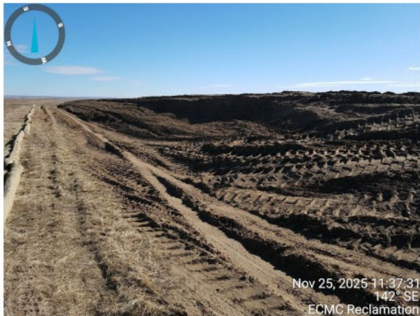
Photo 6. Photo taken from the northern perimeter of location, facing East. Photo illustrates the topsoil stockpile that remains unconsolidated and will be stabilized per the Operator plan.
