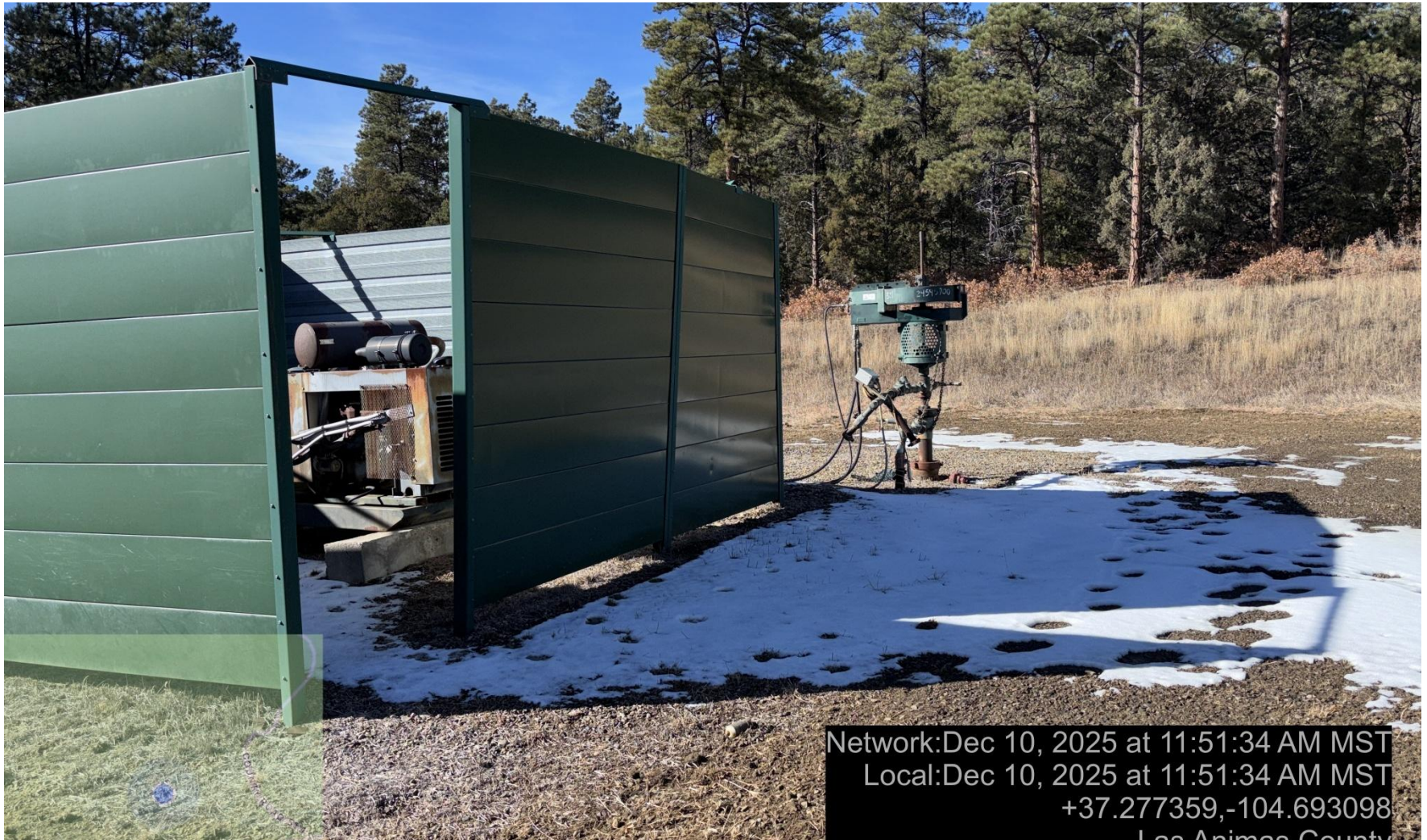
PHOTO 3: WELLHEAD AND EQUIPMENT.
