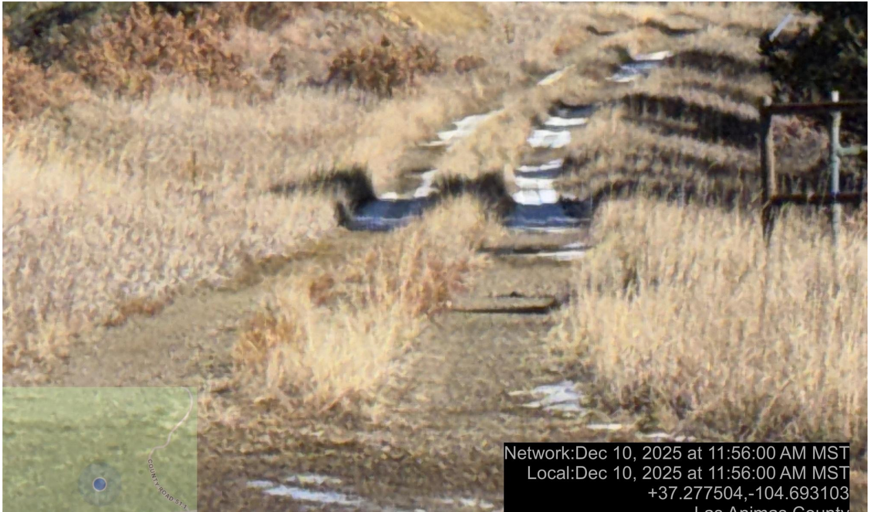
PHOTO 4: WHEN THE WEEDS ON LOCATION WAS MAINTAINED THE TALL DRY WEEDS DOWN THE SENTERLINE OF THE ROAD SHOULD HAVE BEEN MAINTAINED ALSO.
