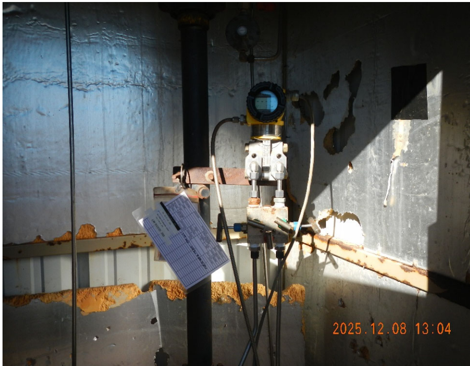
3. Gas Meter inside Meter Shed.
