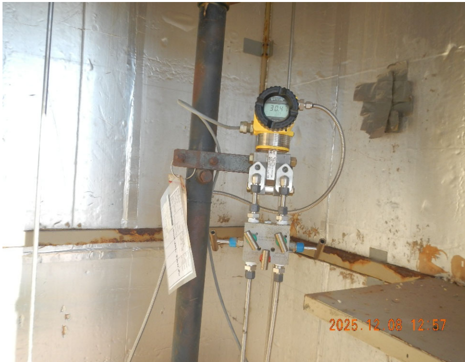
3. Gas Meter inside Meter Shed.
