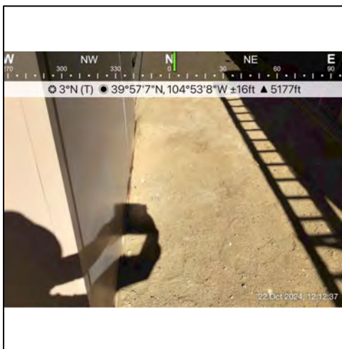
P5 - Clean backfill and road base have been emplaced to match the existing contour of the Site.
