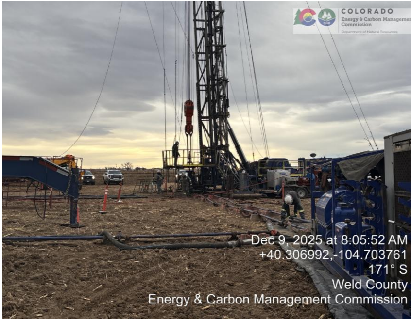
Photo 1 well head and equipment
