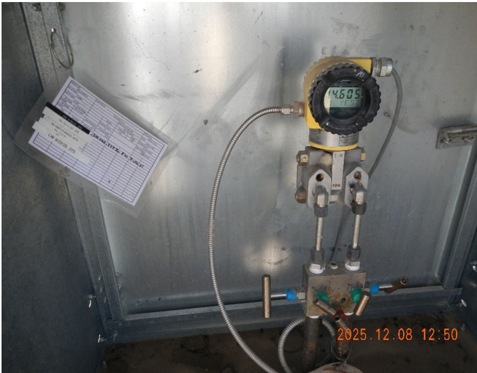
3. Gas Meter inside Flowline mounted Meter Box.
